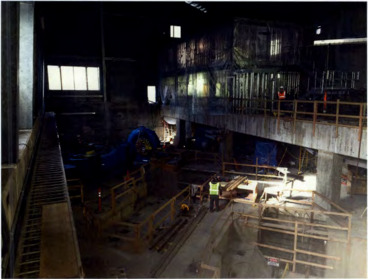
Figure 10. Powerhouse Interior, The powerhouse crane's 45 ton hoist was certified. NAES began placing electrical gear on turbine deck and also set unit 5 spiral case and began alignment. ASRC McGraw Constructors began framing and building out the control room.
