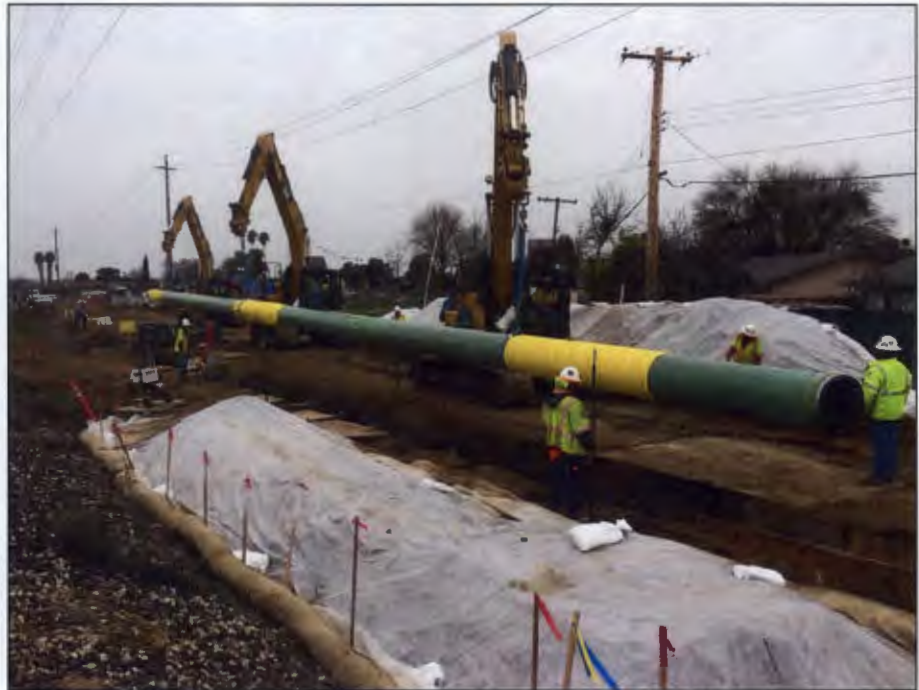
Work on the R-298 Sac RT Relocation Project gets underway in Sacramento.
