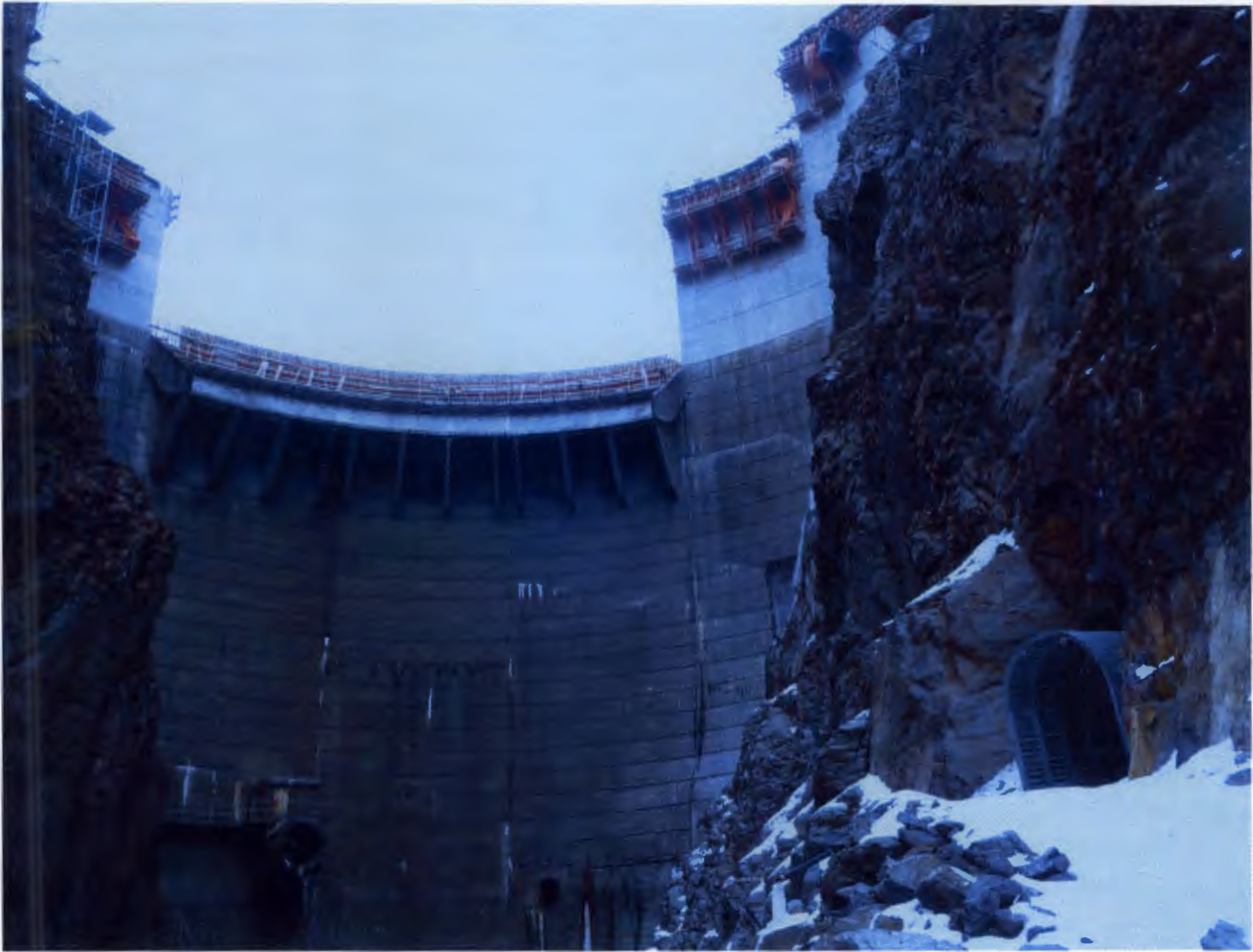
Figure 2. Drainage Tunnel and Scour Wall, AUS divers were on site to work on the dam's sluice gate/trashrack (on the other side of the Howell Bunger Valve pictured above).
