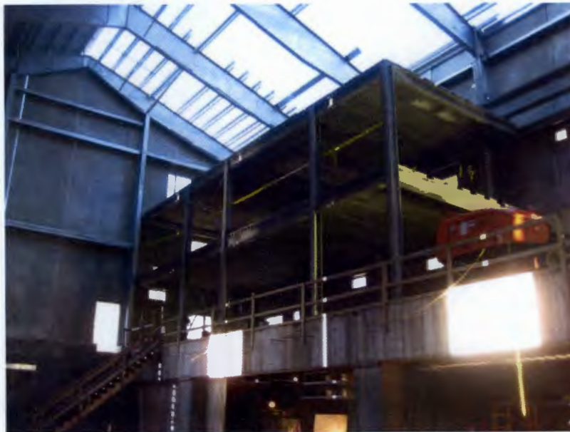
Figure 1: Powerhouse Control Room and Offices
