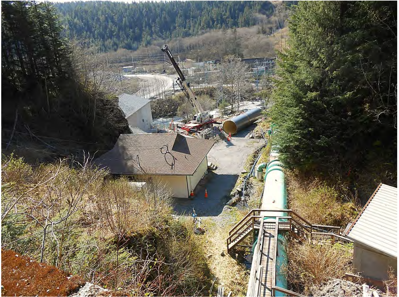
Figure 6. Lower Portal Area, Barnard installed the new penstock from the turbine inlet pipes up to the water treatment plant access road.
