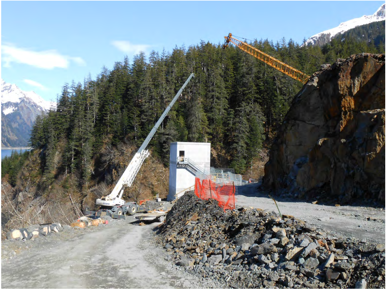
Figure 4. Gate House Location, Barnard, NAES, and Schmolk began the inside buildout of the gate house.
