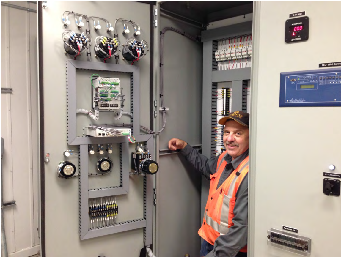
Switchyard control panels fabricated by Bruce Belley, CBS Electric Department employee, for the Blue Lake Expansion project.
