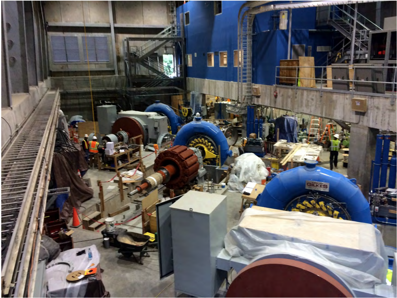
Figure 8. Powerhouse Interior, NAES performed the following tasks related to the turbine generator installation: Unit 3 is fully installed and ancillary mechanical and electrical equipment is 50% complete, Unit 5 is 70% installed and ancillary equipment is 10% complete, Unit 4 is 40% installed and ancillary equipment is 10% complete and continued to install control cables.
