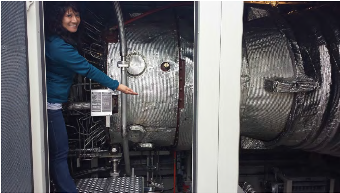
Figure 1. Titan 130 Diesel Turbine
