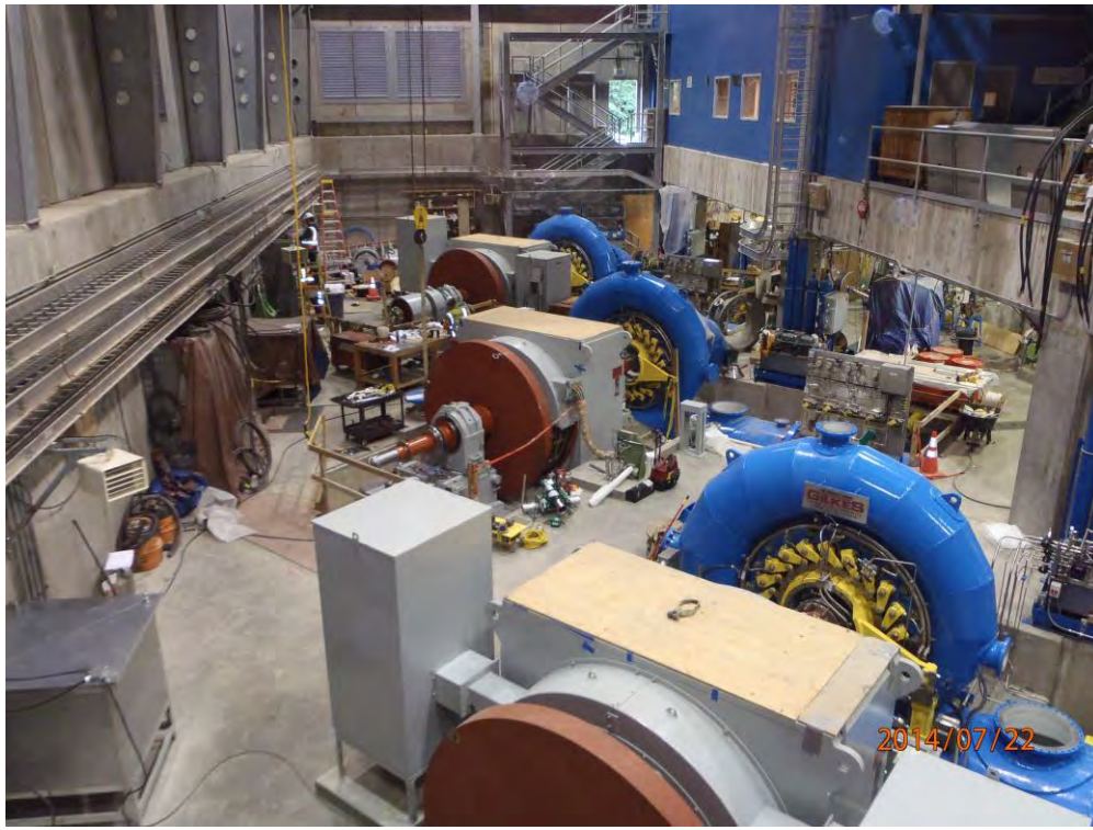
Figure 3: Powerhouse Turbine Floor
