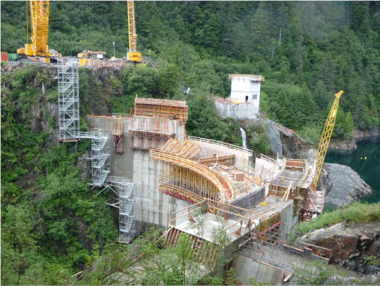
Figure 3. Intake Portal and Right Abutment, The new intake structure is 90% submerged. Crux completed all but 6 curtain grout holes on the right abutment.
