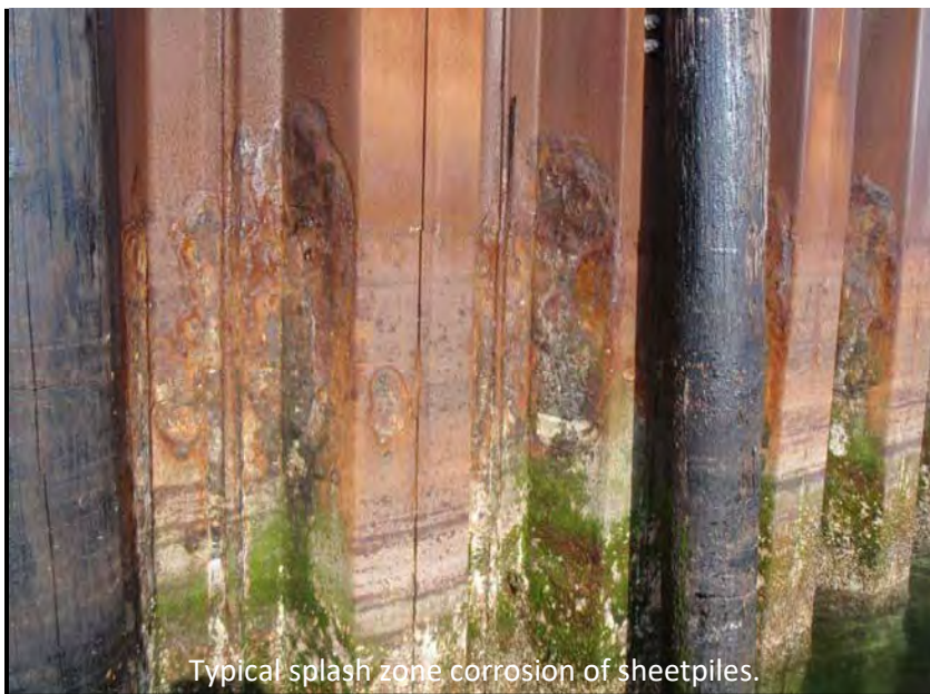
Figure 2 – Splash Zone Corrosion of Sheetpile – July 2011
