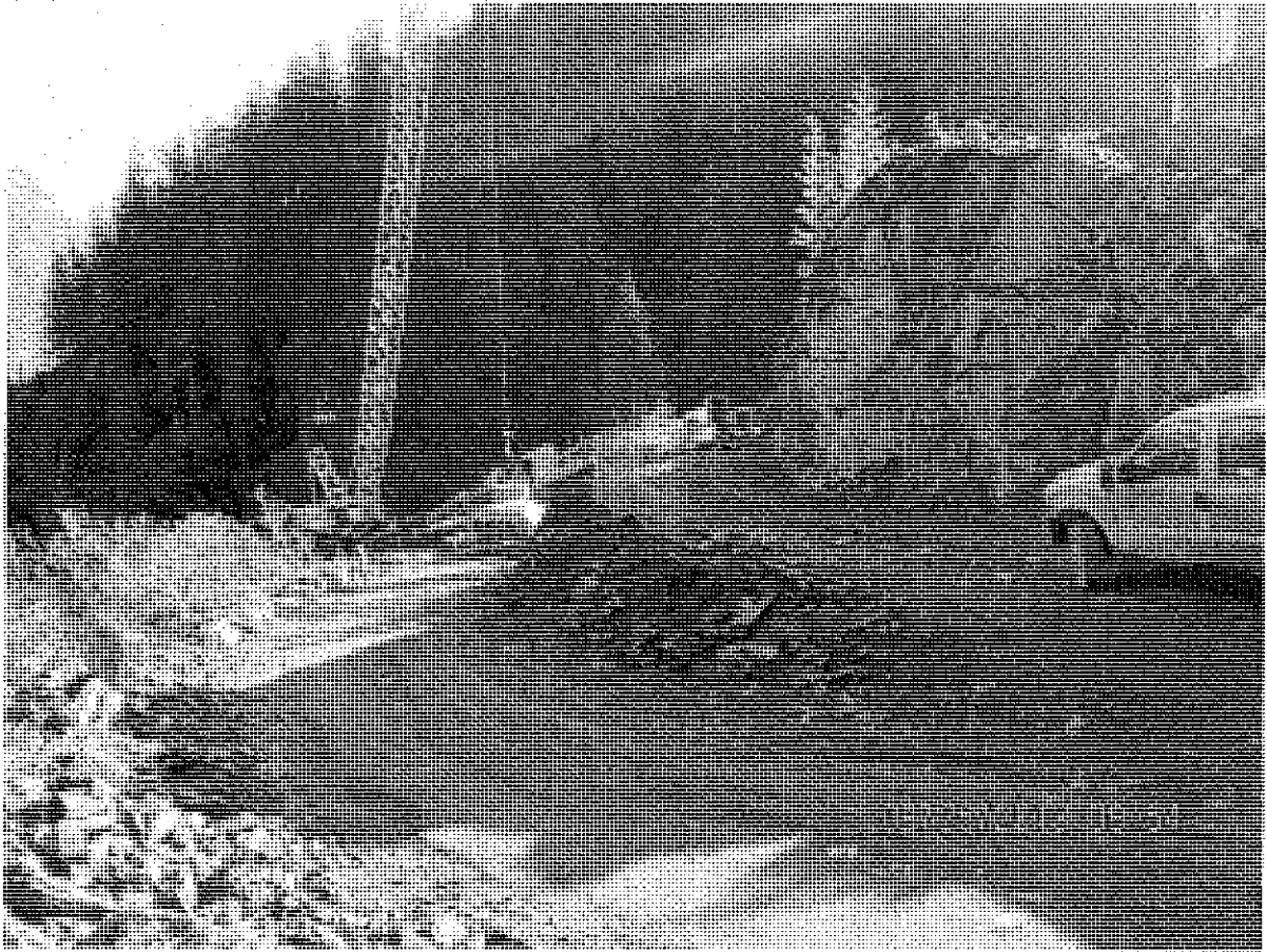
Figure 4. Gate House Location, Barnard continued construction of the gate chamber. The floor and walls have been placed. Forms are being installed to place the crown.
