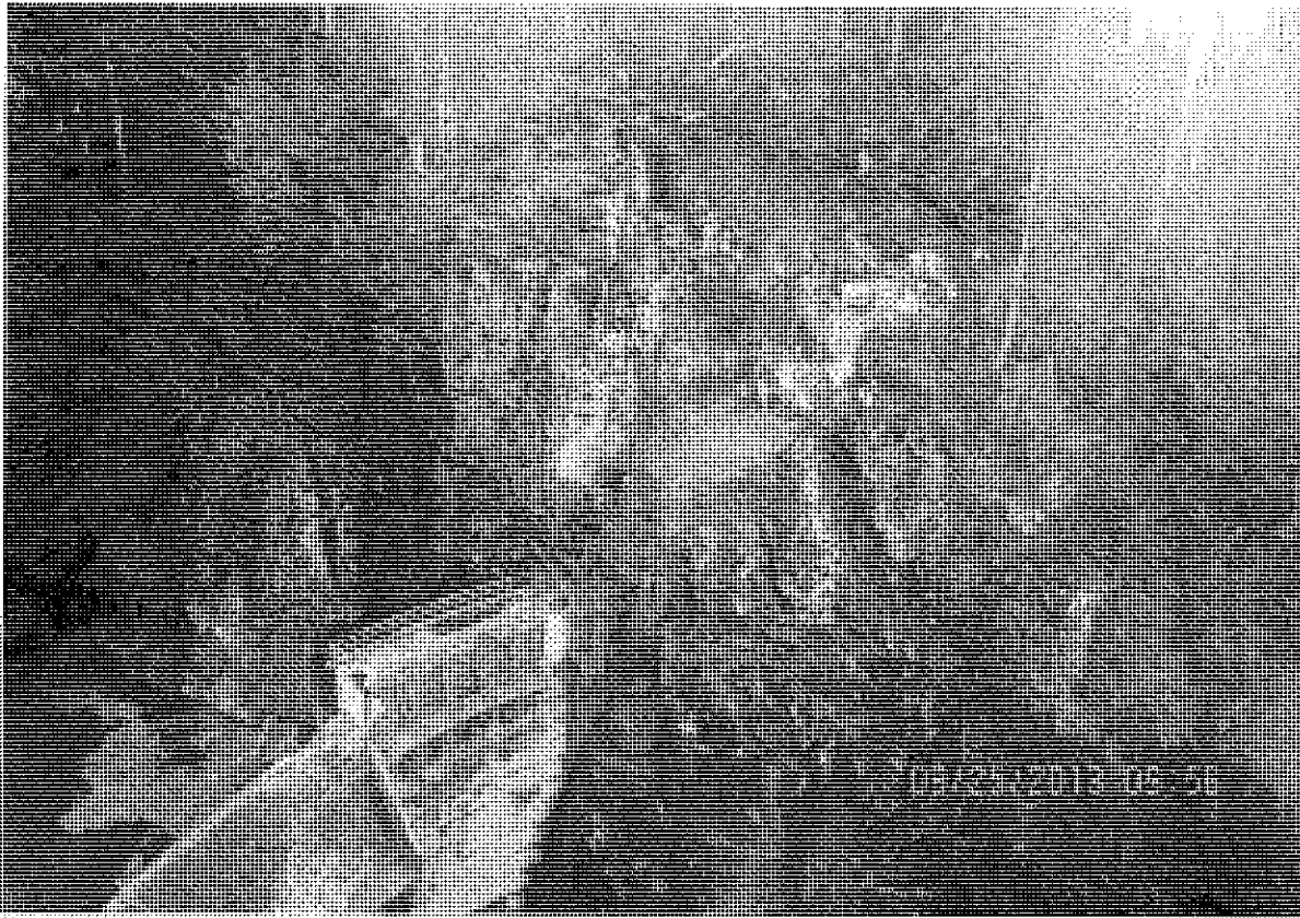
Figure 1. Dam and Left Abutment Area, Harvard continued placing concrete blocks to raise the dam. A total of two 18-ft high blocks are complete on the dam next to the left abutment.
