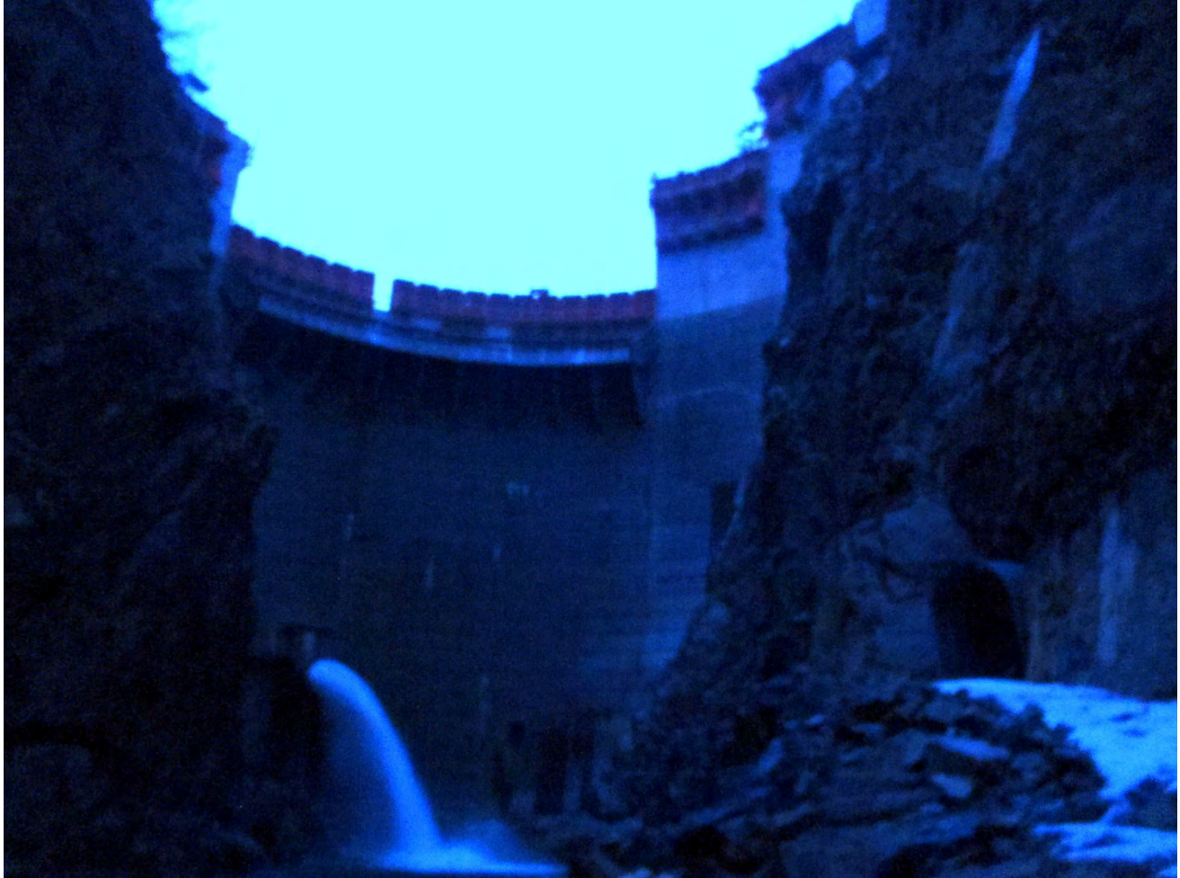
Figure 2. Drainage Tunnel and Scour Wall, A change work directive was issued to provide a dam release pipe in the dam extension above the existing spillway. The pipe is on site and will be installed in the new dam in April.
