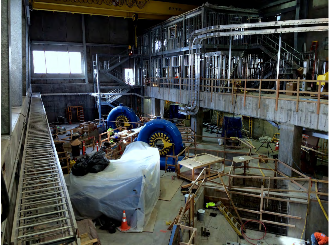
Figure 9. Powerhouse Interior, Schmolk began the powerhouse mechanical rough-in. Completed final alignment of BLU unit 5 turbine spiral case and grouted in place. Placed BLU unit 5 turbine draft tube. Completed final alignment of BLU-5 sole plates and epoxy grouted the anchor bolts. NAES continued with installation of conduit and cable tray in powerhouse and installed conduit for lighting and plant services. ASRC continued framing and building out the control room.
