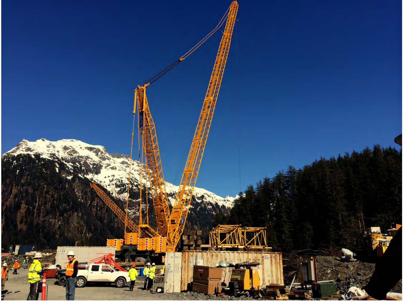
Figure 5. Dam Staging area, a new smaller 150 ton Liebherr crane was set up to assist with the dam raise.
