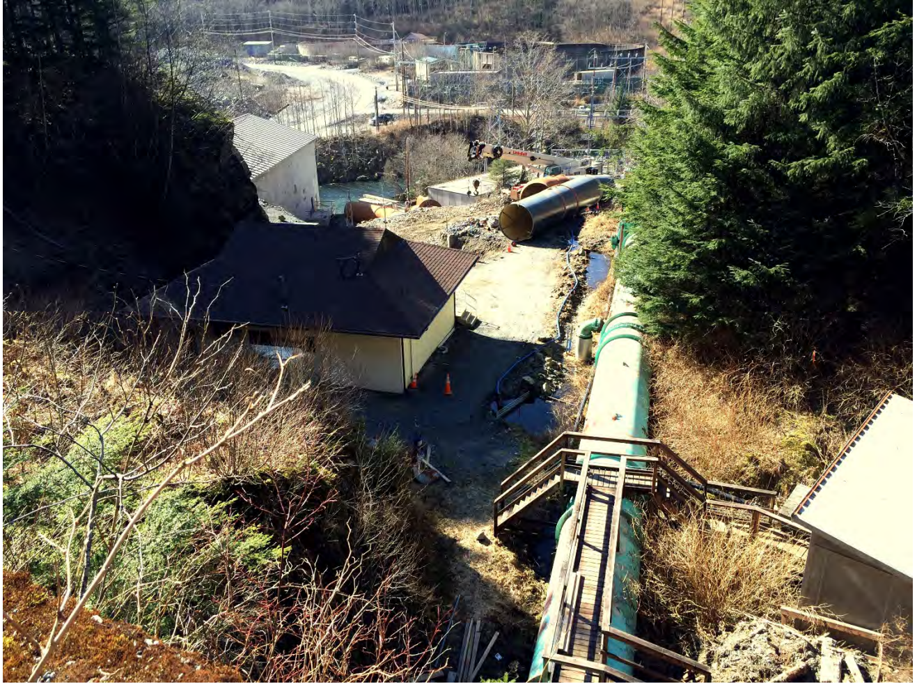
Figure 6. Lower Portal Area, Staged penstock segments at powerhouse. Southeast Earthmovers completed excavation for penstock segment 6.
