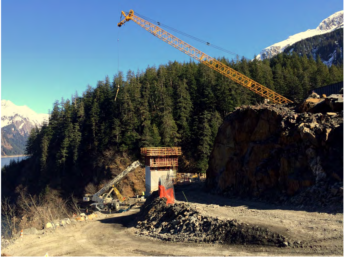
Figure 4. Gate House Location, Removed final forms from gatehouse. Concrete for this structure is complete.
