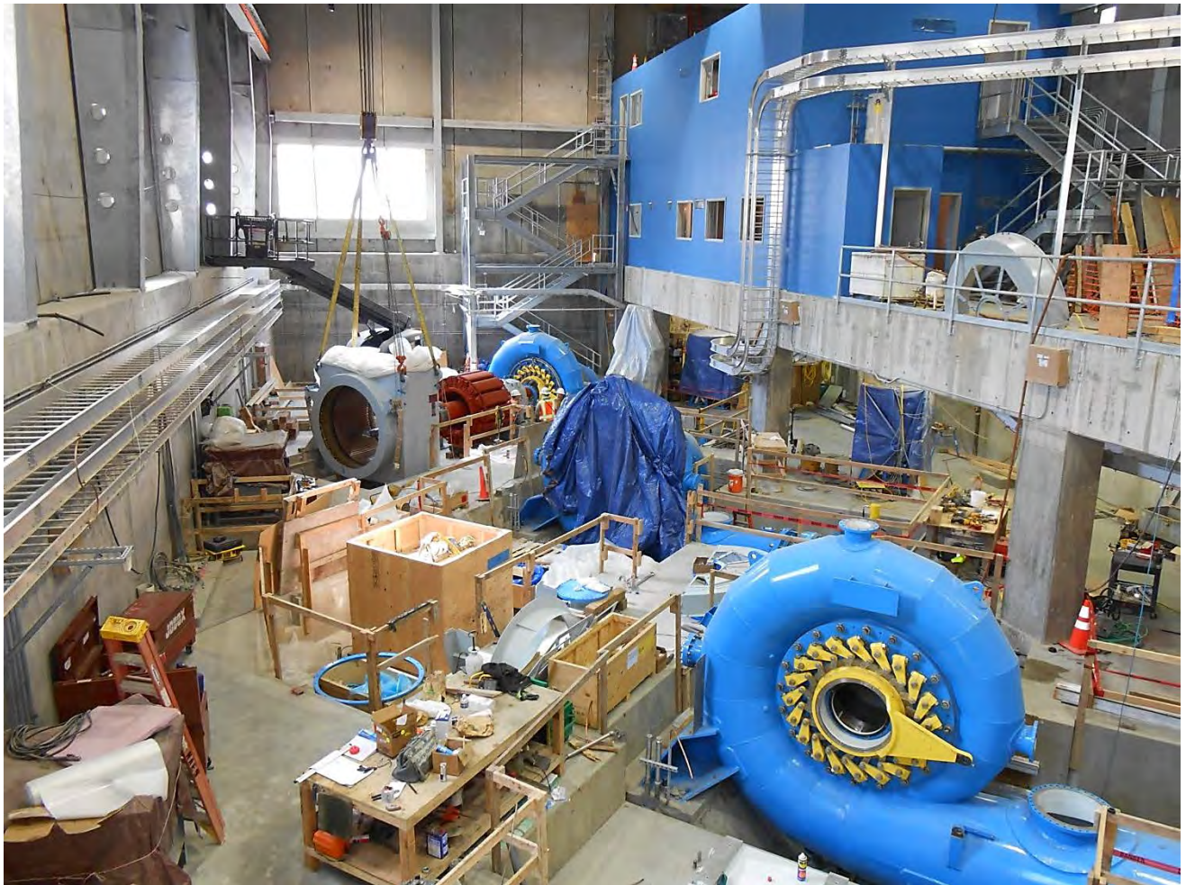
Figure 8. Powerhouse Interior, ASRC completed 90% of the control room buildout. NAES placed secondary concrete around BL5&3 draft tubes, completed alignment of all 3 turbine spiral cases, set all 3 turbine inlet valves, completed alignment of BL5&3 generator sole plates and installed generator stator, rotor, and bearings on BL5. NAES also continued with installation of conduit and cable tray in and outside the powerhouse and began installing electrical panel boards.
