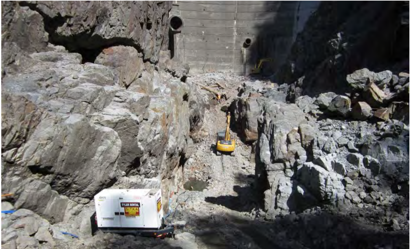
Figure 2. Drainage Tunnel and Scour Wall, Plunge pool was dewatered for scour wall installation. Crux arrived on site to begin curtain grouting and scour wall construction.
