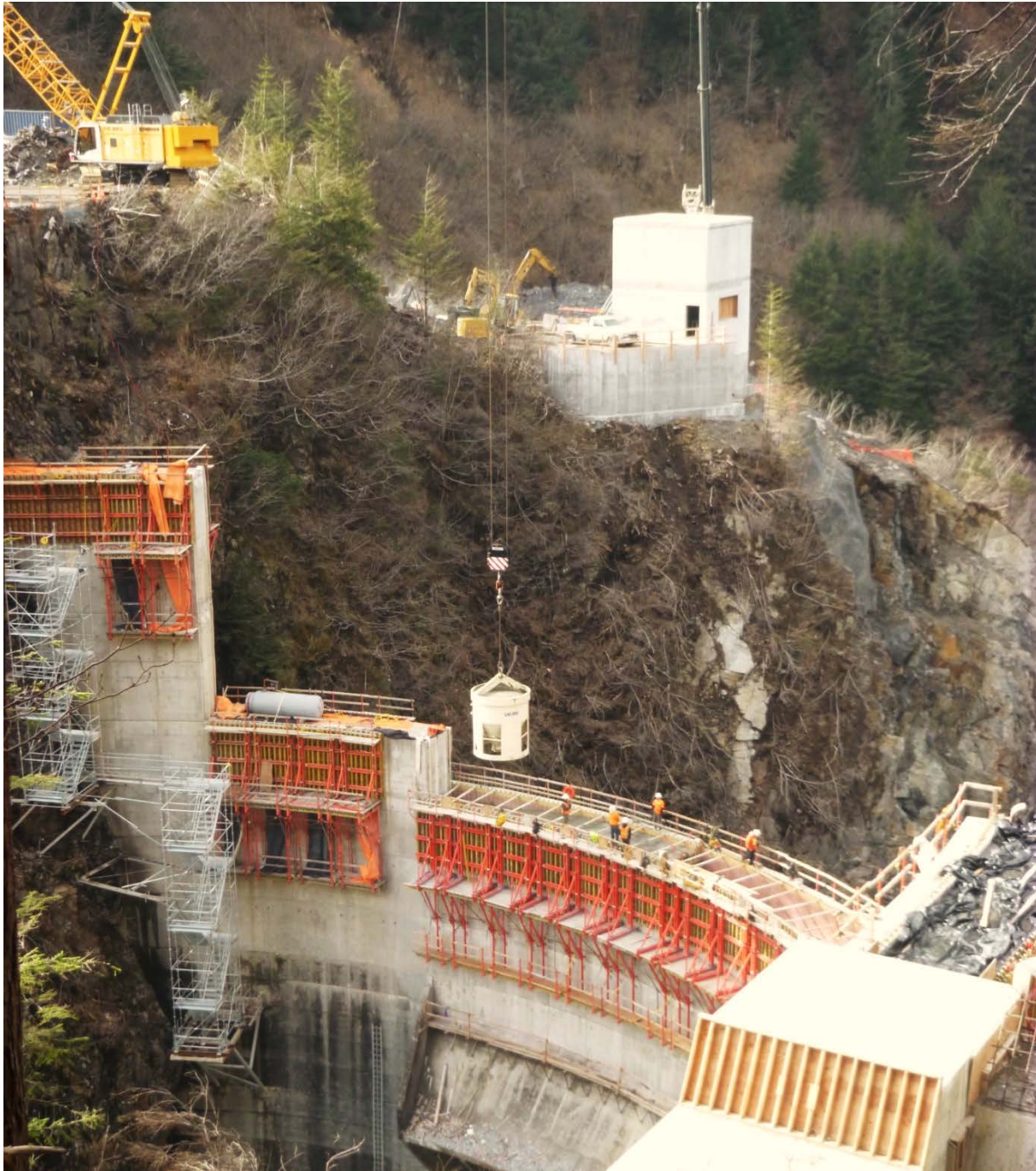
Figure 3. Intake Portal and Right Abutment, Barnard completed the intake rock bolting and the intake chamber concrete work. They have also set the trash rack frame and begun work on the intake structure concrete. (Not seen in this picture due to the new height of the dam.)
