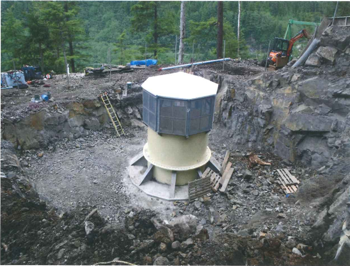
Figure 6. Surge Chamber Top Portal, The small structure over the surge shaft is complete.
