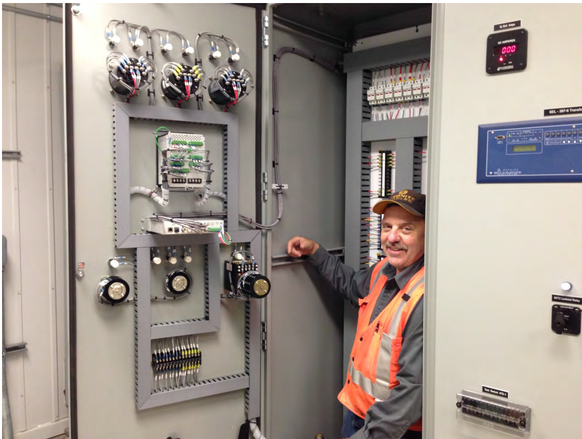
Switchyard control panels fabricated by Bruce Belley, CBS Electric Department employee, for the Blue Lake Expansion project.
