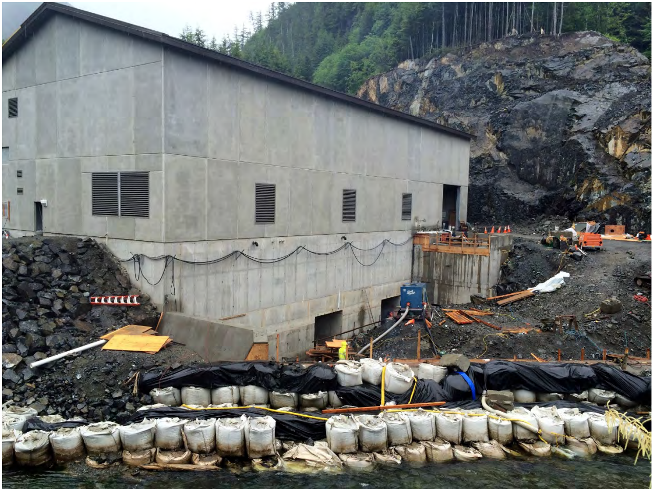
Figure 7. Powerhouse Site, AMCL continued work on the raw water intake and after bay.
