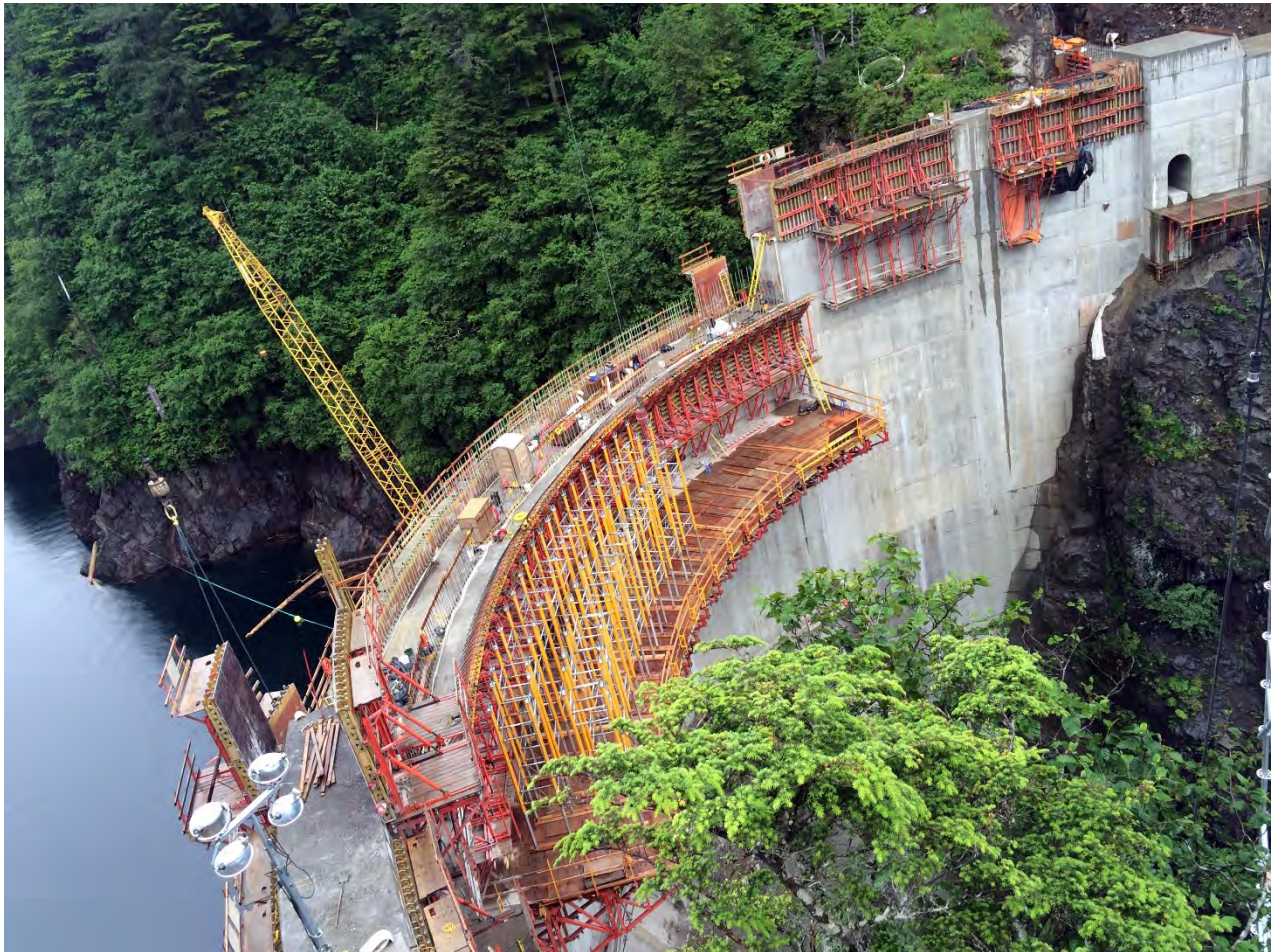
Figure 1. Dam and Left Abutment Area, Barnard showed good progress on the dam construction completing 8 block placements. To date 51 of 53 blocks placed on the Dam Raise. In June Barnard started work on the spillway section of the dam, which is the most complicated formwork for the dam raise. Eight of 9 placements completed on the Left Abutment and Cutoff Wall.
