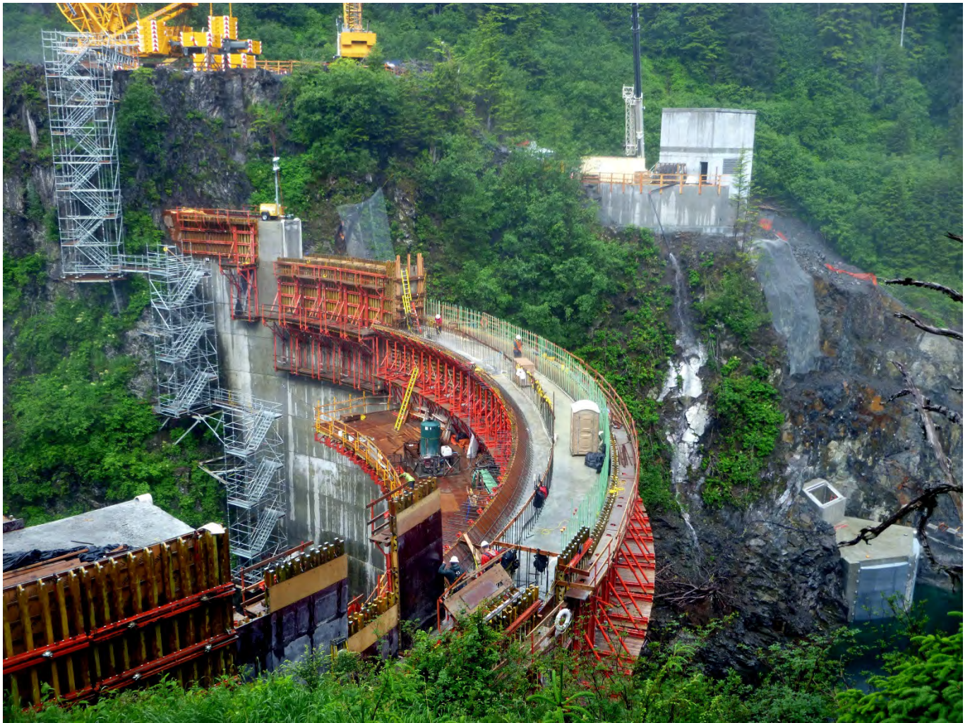
Figure 3. Intake Portal and Right Abutment, Barnard completed the new tunnel intake structure on time, Project Milestone No. 4. The new intake structure is now 50% submerged.
