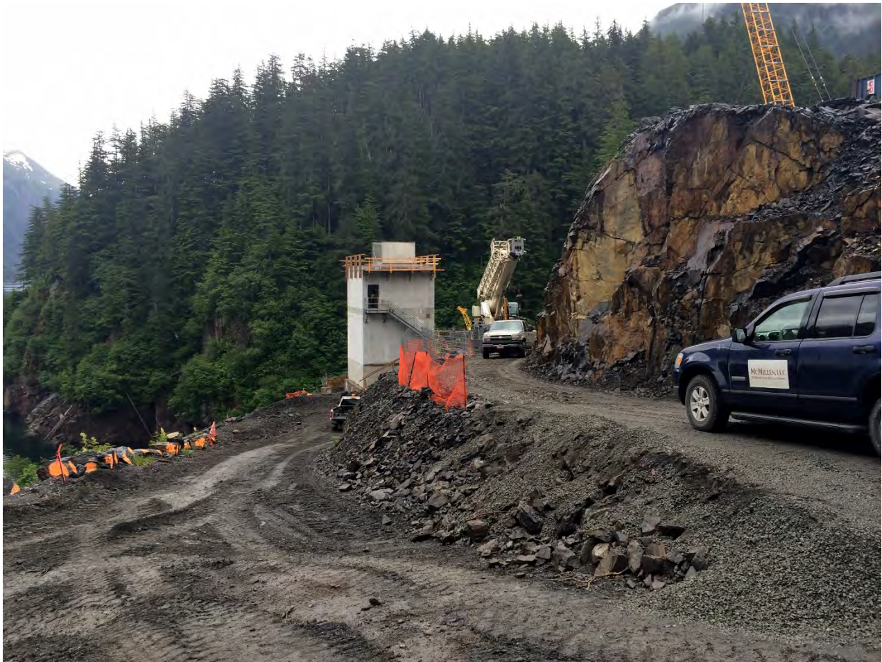
Figure 4. Gate House Location, Barnard completed the roof and roof hatch at the Gate House.
