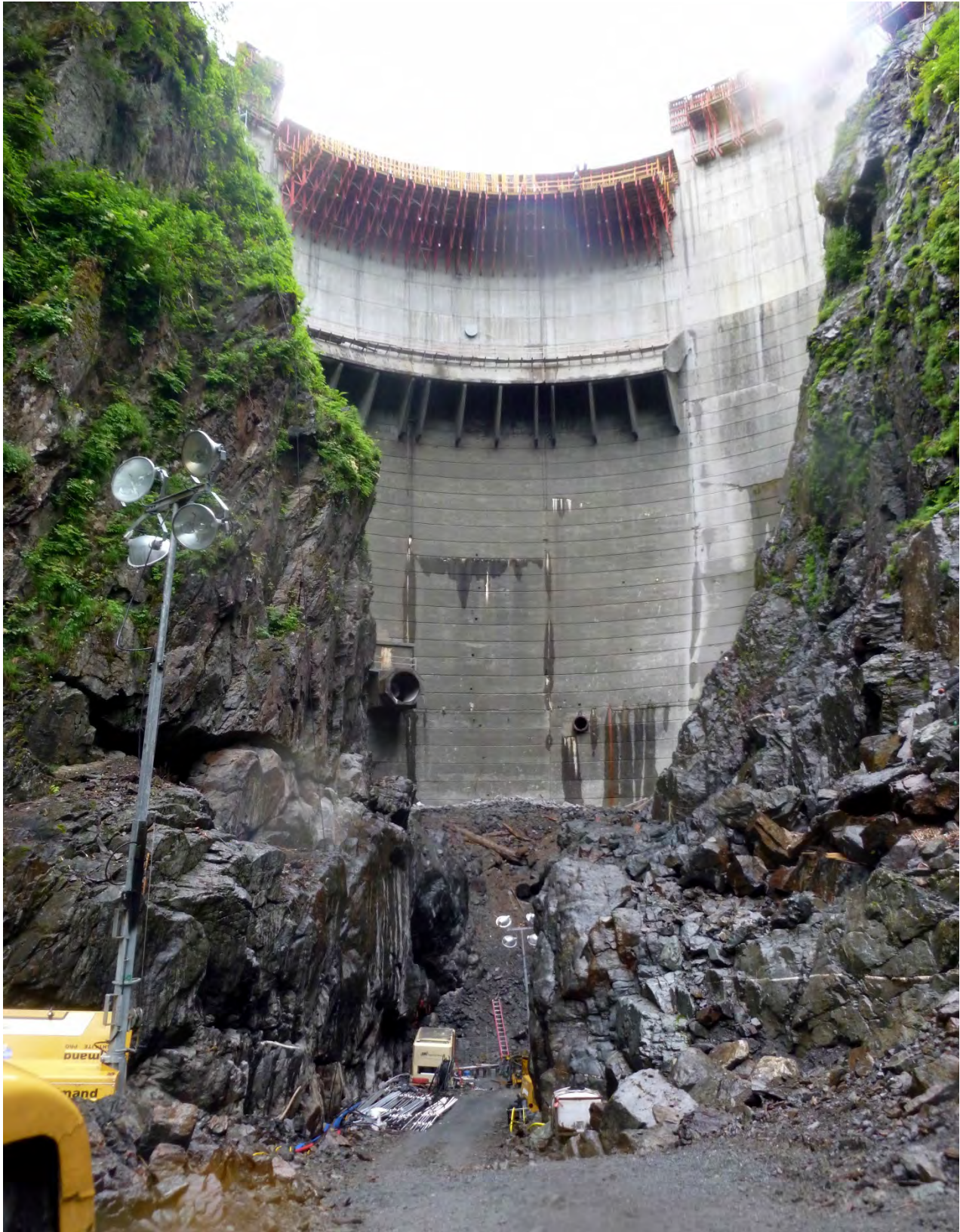
Figure 2. Drainage Tunnel and Scour Wall, Crux completed all of the micro piles required by the contract and began drilling for the placement of rock anchors.
