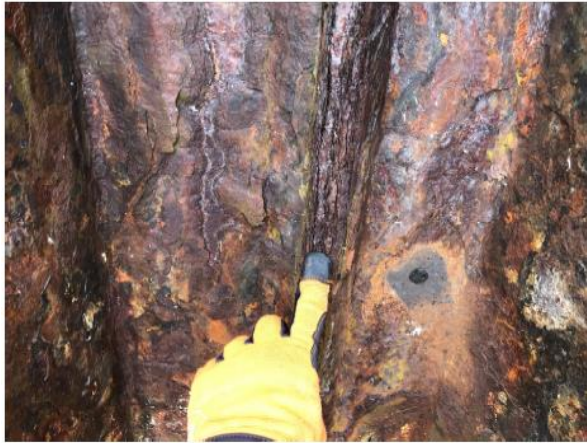
Figure 2 - Sheet Pile Corrosion in Splash Zone, July 2021
