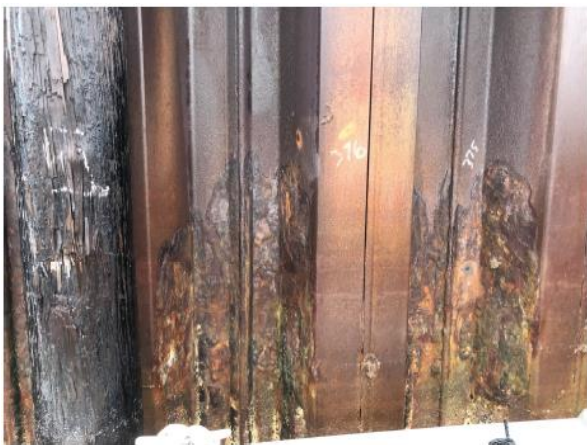
Figure 3- Sheet Pile Corrosion in Splash Zone, July 2021
