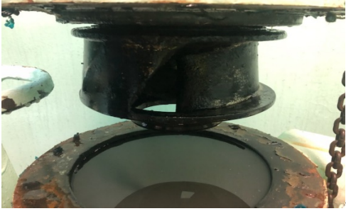
- This photo shows the impeller free of wiper seals
