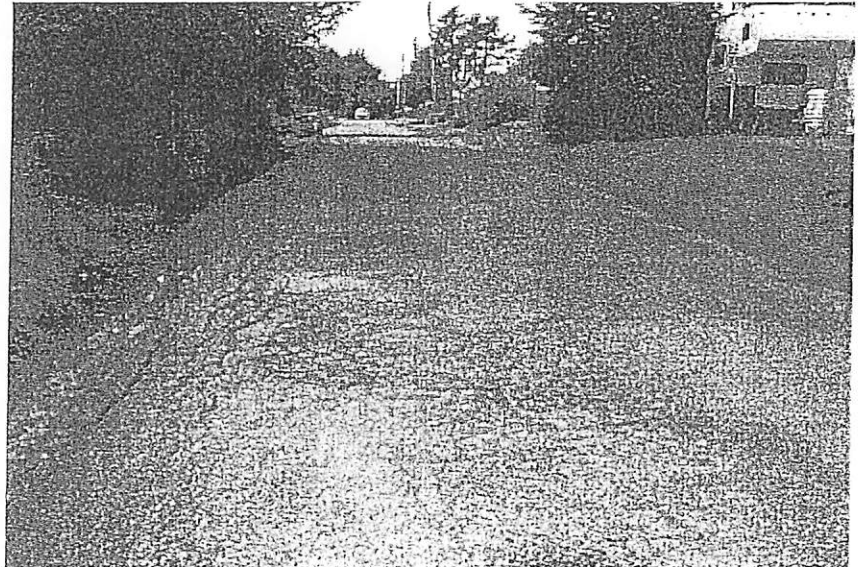
An example of poor asphalt condition due to subgrade issues. This is indicative of the condition of many municipal roads in Sitka.
