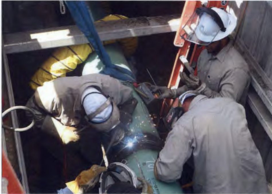
A crew performs a tie-in weld at a Barnard PG&E Alliance project site.
