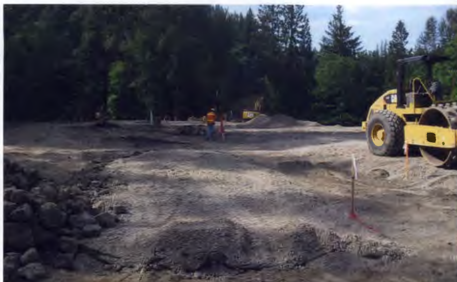
Crews grade the public parking area, which receives up to 2 million visitors annually.
