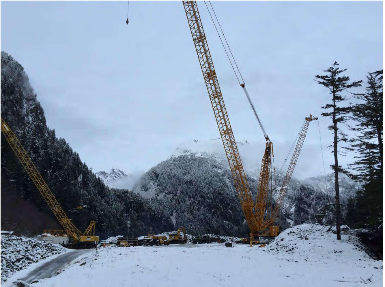
Figure 4. Dam Staging area, In preparation for crane demob, the staging area has been cleared.
