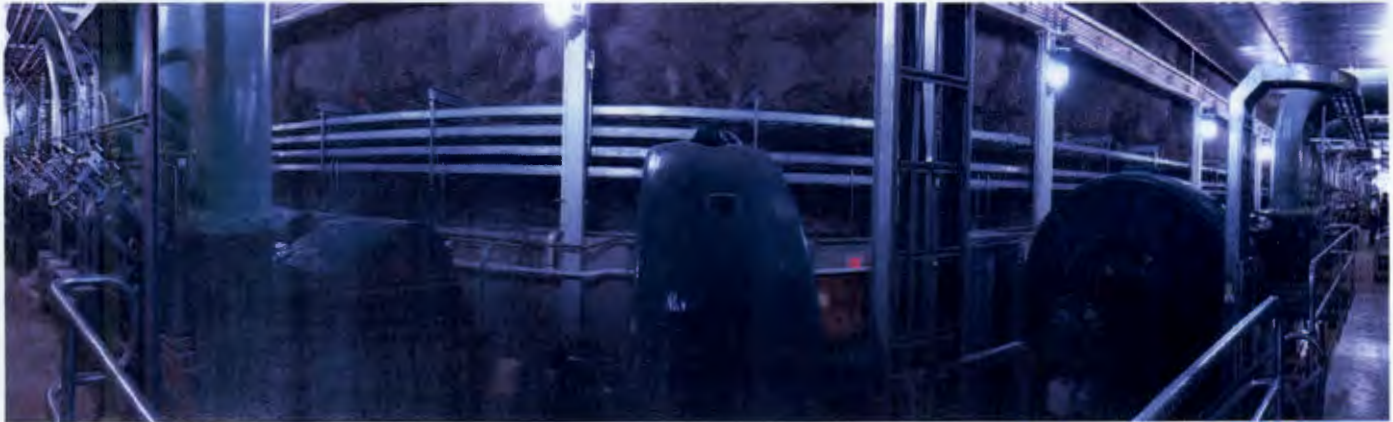
A look at the Plant 1 Powerhouse Pelton units. Needle valves and controls are on the left and Units 2 and 3 and testing personnel can be seen on the right.
