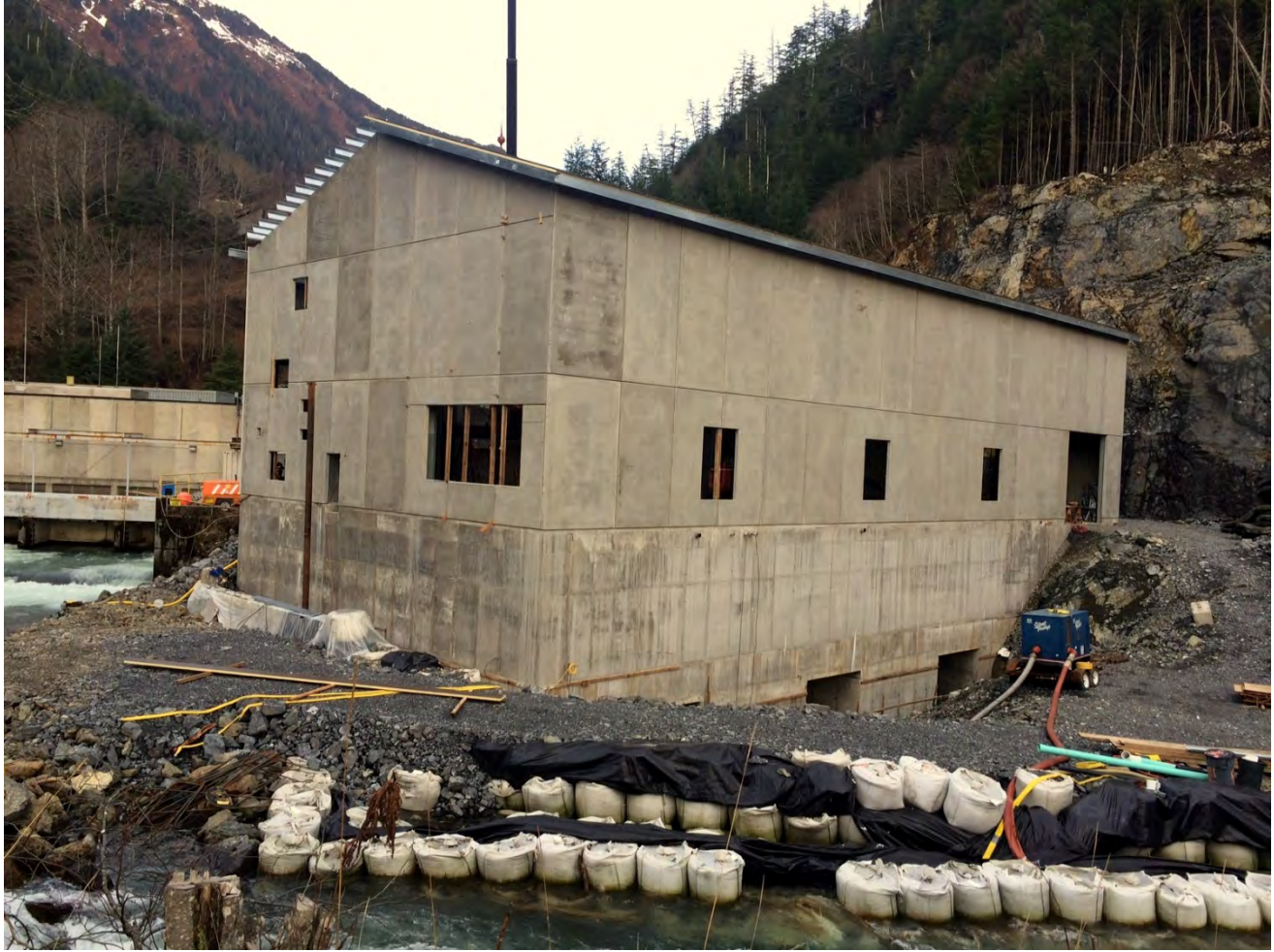
Figure 7. Powerhouse Site, ASRC McGraw Constructors (AMCL) completed the installation of the concrete wall panels and began the installation of the roof panels.
