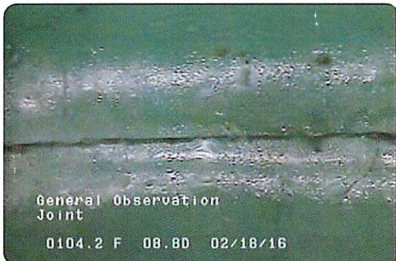
General Observation at 104.2 feet | Joint
