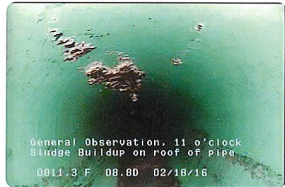
General Observation at 011.3 feet, 11 o'clock | Sludge Buildup on roof of pipe
