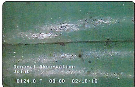
General Observation at 124.0 feet | Joint
