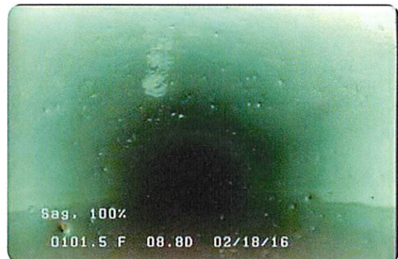
Sag at 067.3 feet, continuous for 34.2 ft, 100%
