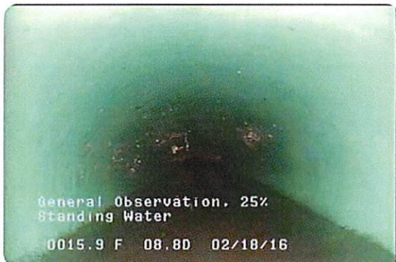
General Observation at 015.9 feet, 5-7 o'clock, 25% | Standing Water
