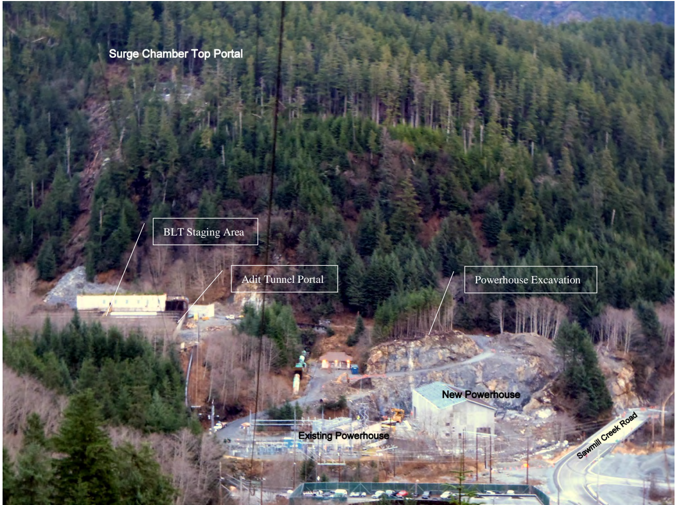
Figure 9. Lower Project Site, Southeast Earthmovers (SEEM) continued excavation on the new powerhouse access road.
