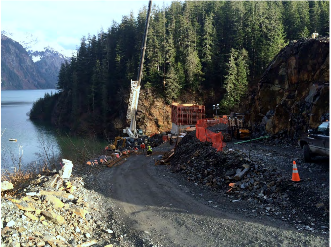
Figure 4. Gate House Location, Barnard made a gate house concrete floor placement and began working nightshift in the gate shaft installing gate guides.
