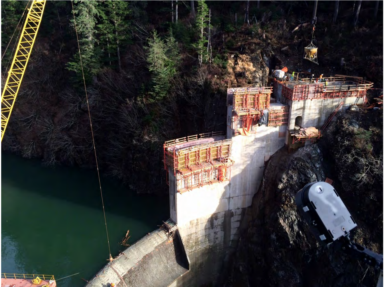
Figure 1. Dam and Left Abutment Area, Barnard made 2 concrete placements at the thrust block, 1 placement at the cutoff wall, and 3 block placements in the main dam near the left abutment. Crux Subsurface also began drilling the dam spillway for installation of keyway rebar.
