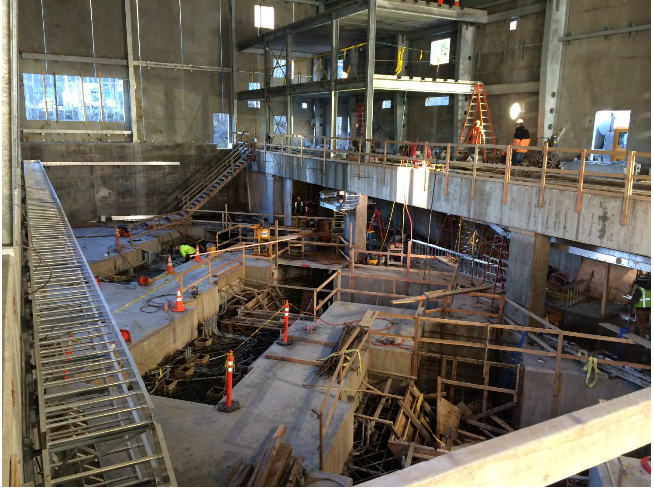
Figure 10. Powerhouse Interior, Powerhouse is now fully enclosed and the control room structure is erected.
