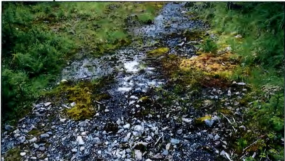
Photo F. Wet spot on mainline road.
