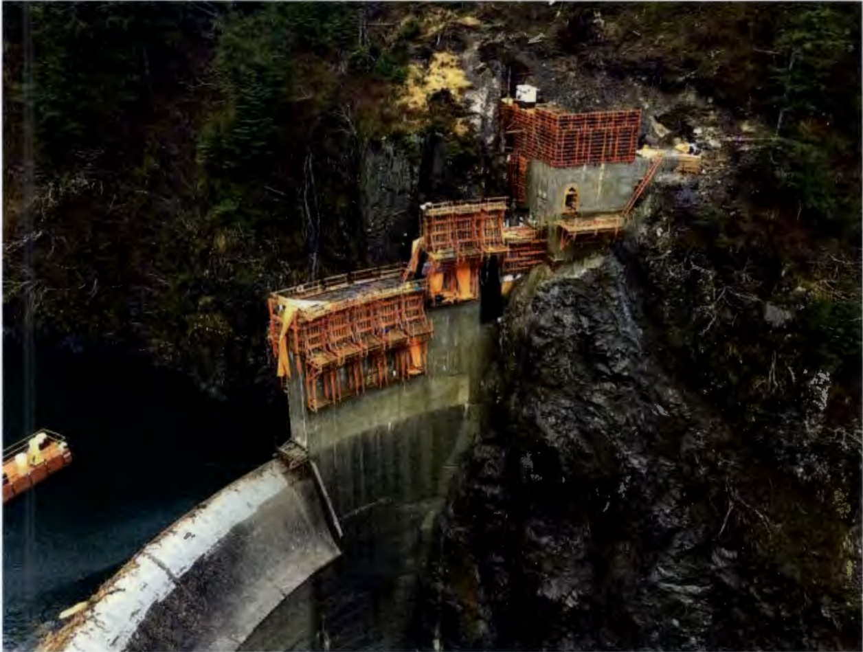
Figure 1. Dam and Left Abutment Area, Barnard made 1 concrete placement at the thrust block, 1 placement at the cutoff wall, and 3 block placements in the main dam near the left abutment. Barnard also prepped the spillway.
