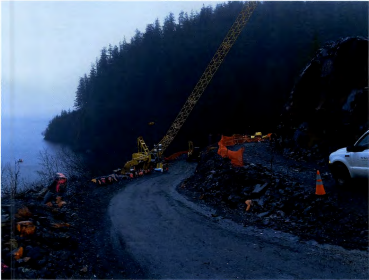
Figure 4. Gate House Location, Barnard completed the last concrete placement in the intake tunnel gate shaft.
