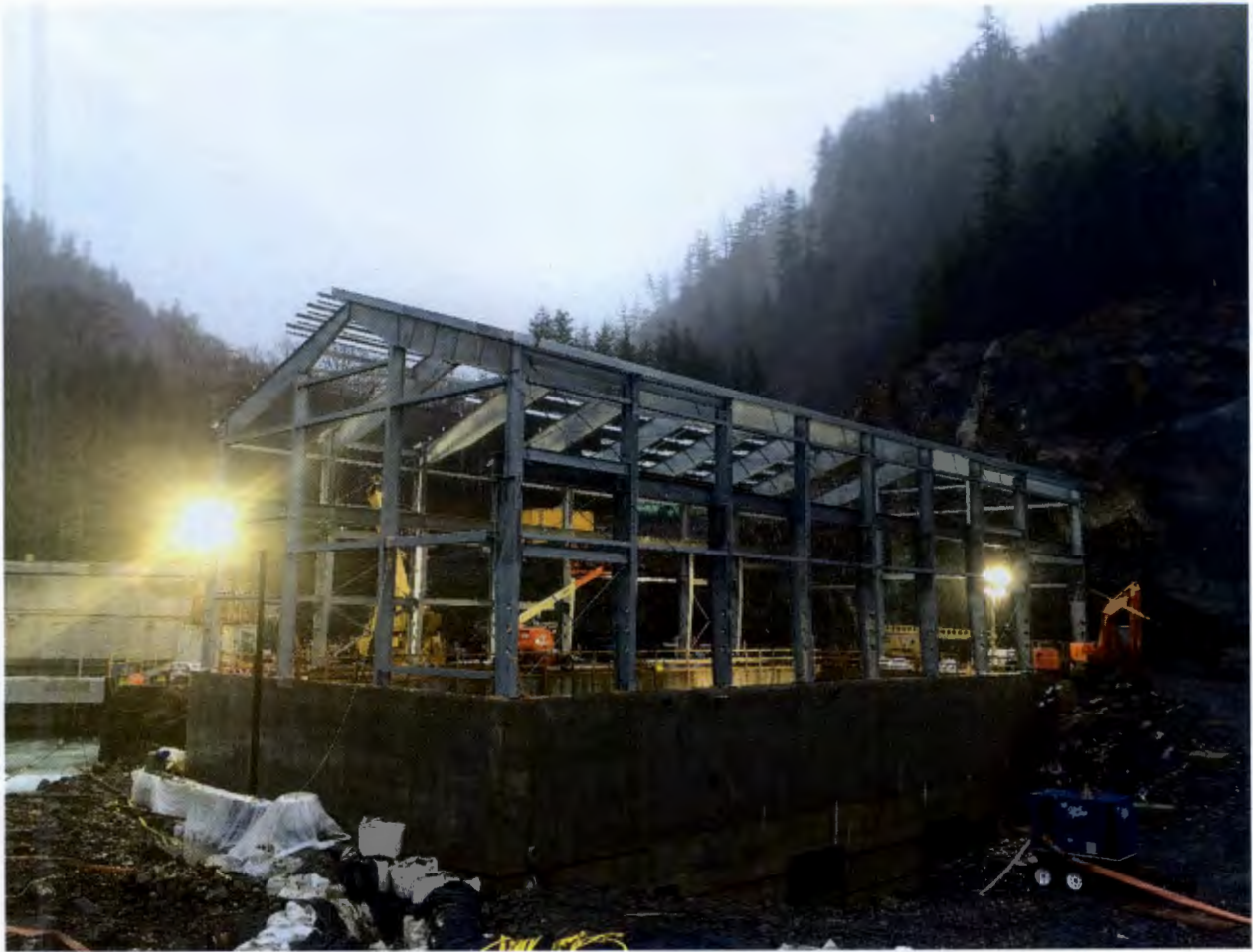
Figure 7. Powerhouse Site, ASRC McGraw Constructors (AMCL) completed the erection of power house steel columns and roof trusses.
