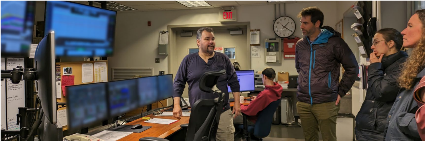
CBS Plant Operators show engineers from the national labs the Supervisory Control and Data Acquisition (SCADA) system at the Blue Lake Powerhouse.
