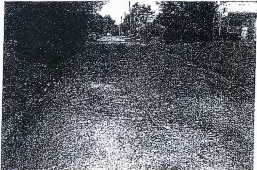
An example of poor asphalt condition due to subgrade issues. This is indicative of the condition of many municipal roads in Sitka.
