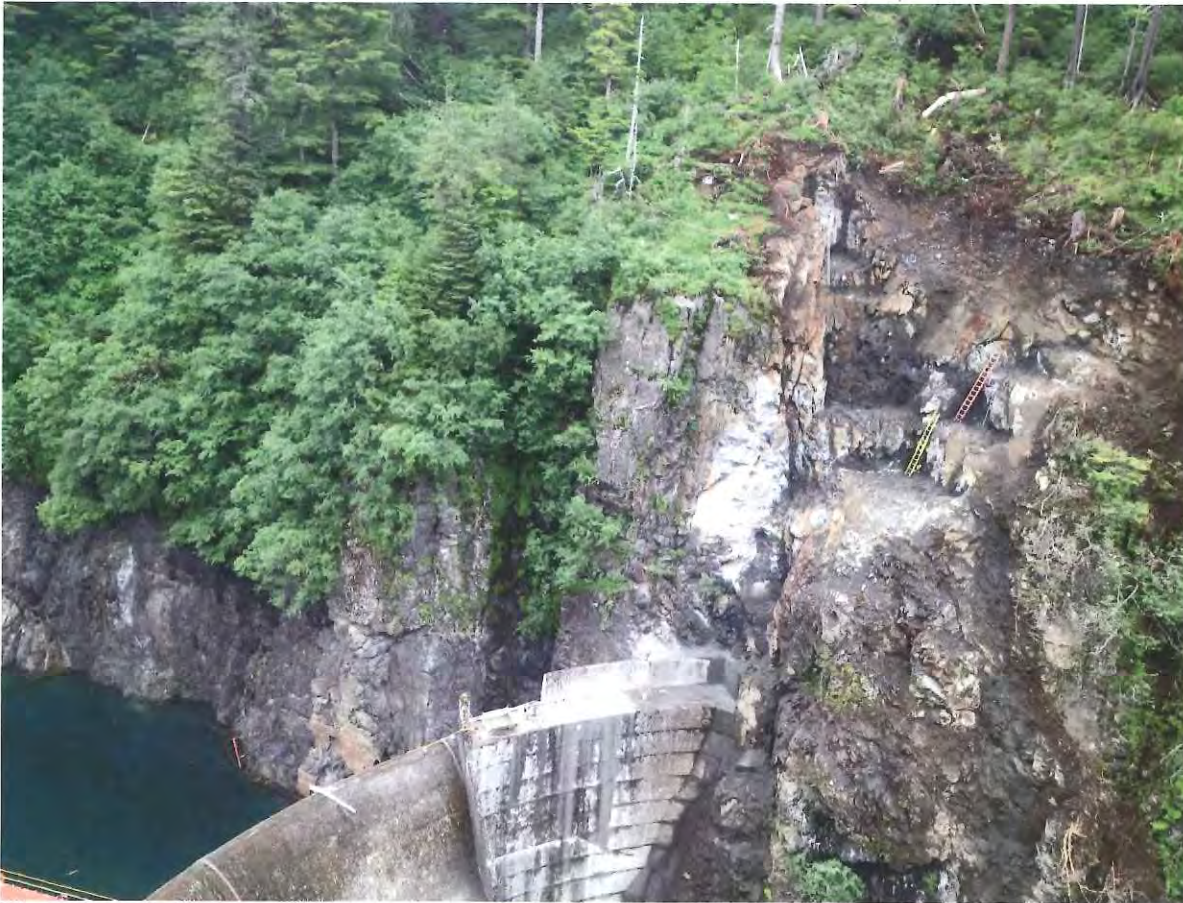
Figure 1. Dam and Left Abutment Area, Blue Lake Tunnelers completed the left abutment thrust block excavation. Work on the keyway began and the first concrete pour was completed on the dam.
