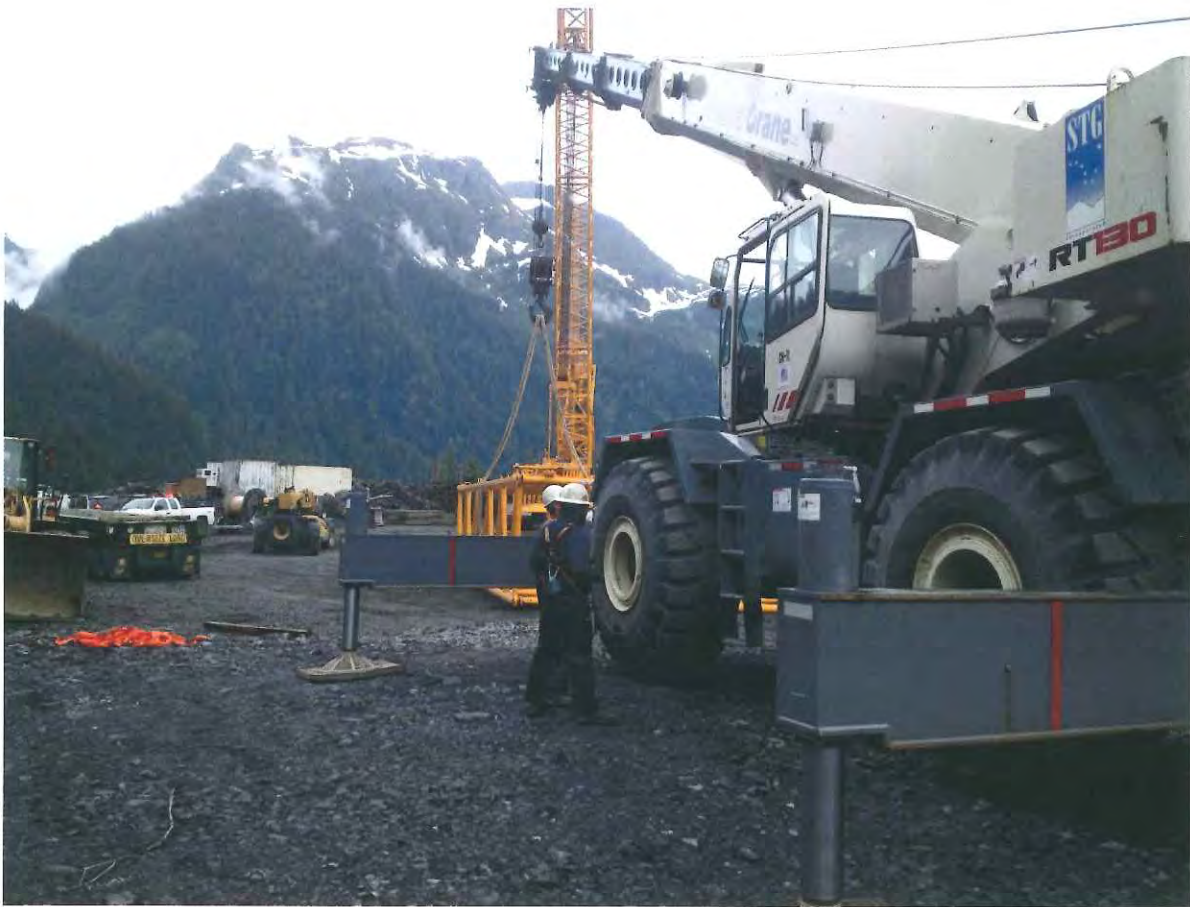
Figure 5. Dam Staging area, The 600 ton crane boom was disassembled to add an additional 40 feet of boom and a new counter weight carriage.
