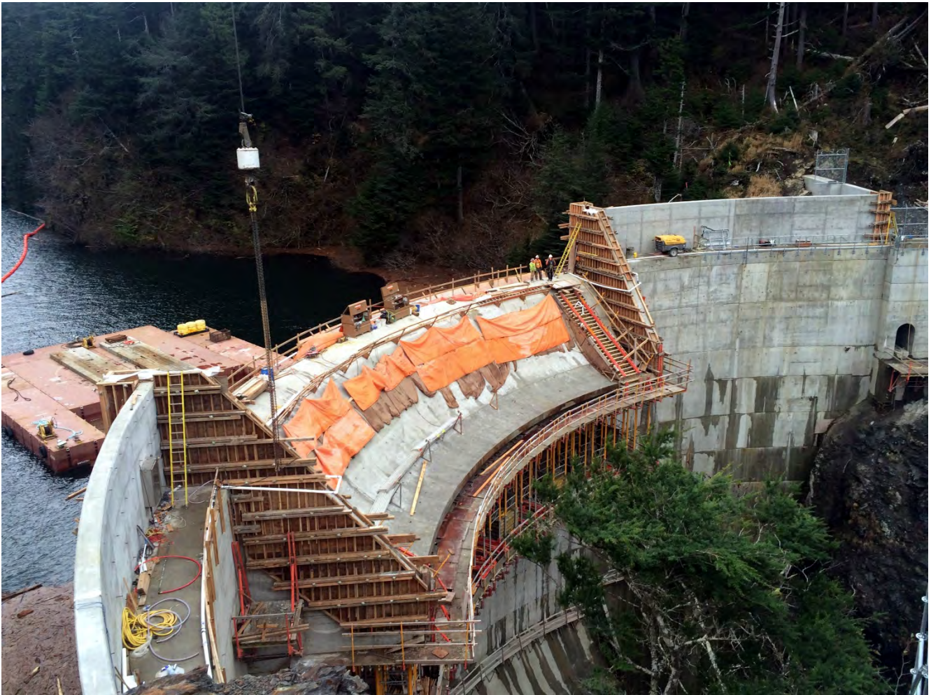
Figure 1. Dam and Left Abutment Area, Barnard crews completed all major concrete placements on the dam and performed dam contraction joint grouting from elevation 403 to 425.
