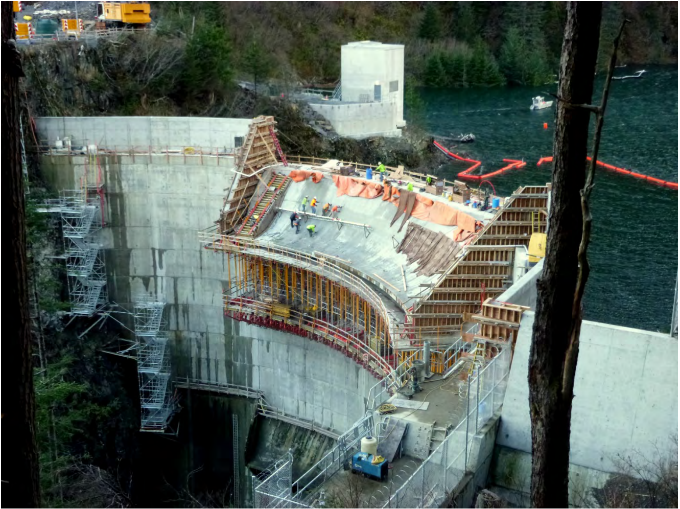
Figure 2. Intake Portal and Right Abutment, The spillway is being sacked and patched as planned.
