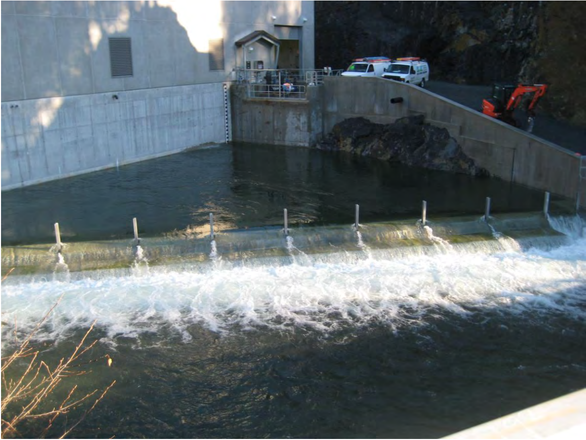
Figure 1: Tailrace during Unit 3 and 5 High Flow Test
