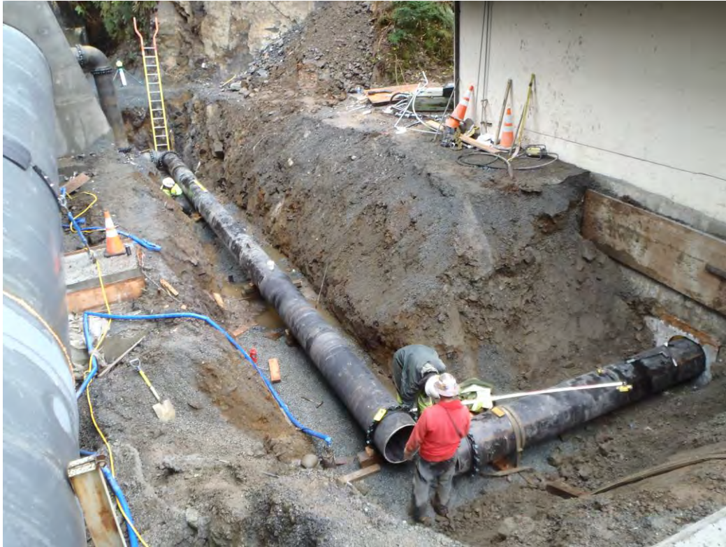
Figure 3: 20" Raw Water Line into WTB
