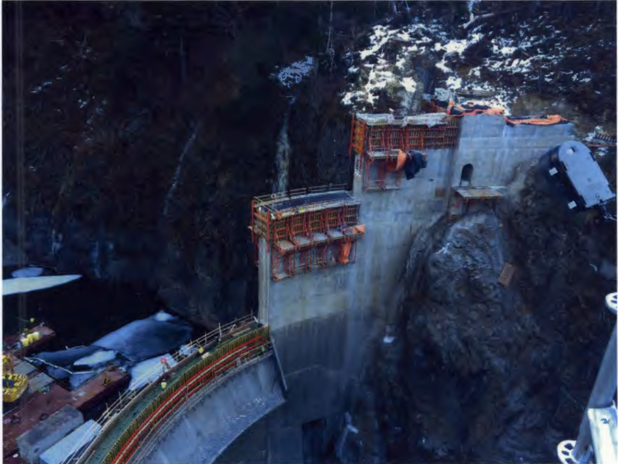
Figure 1. Dam and Left Abutment Area, Barnard completed placing dowels and concrete prep work on existing spillway.
