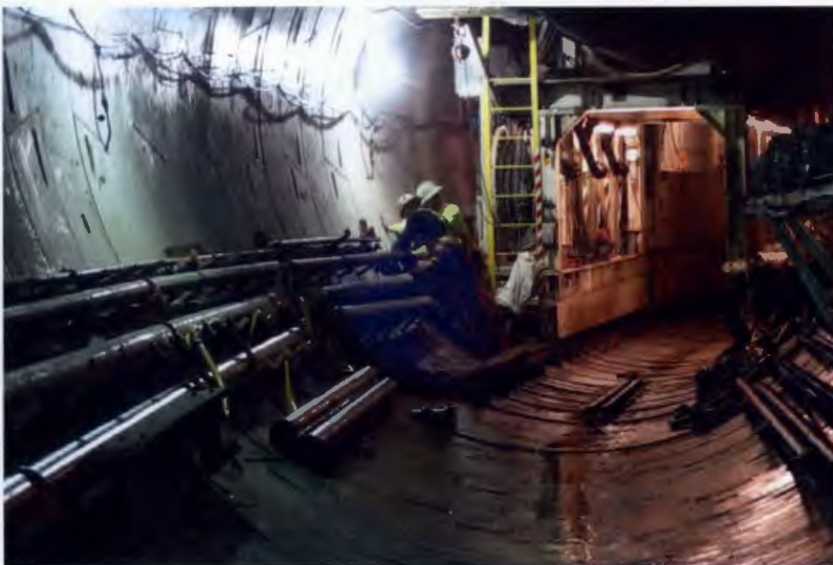
Installing utility pipe in one of the twin tunnels at the Central Subway Tunnel project.
