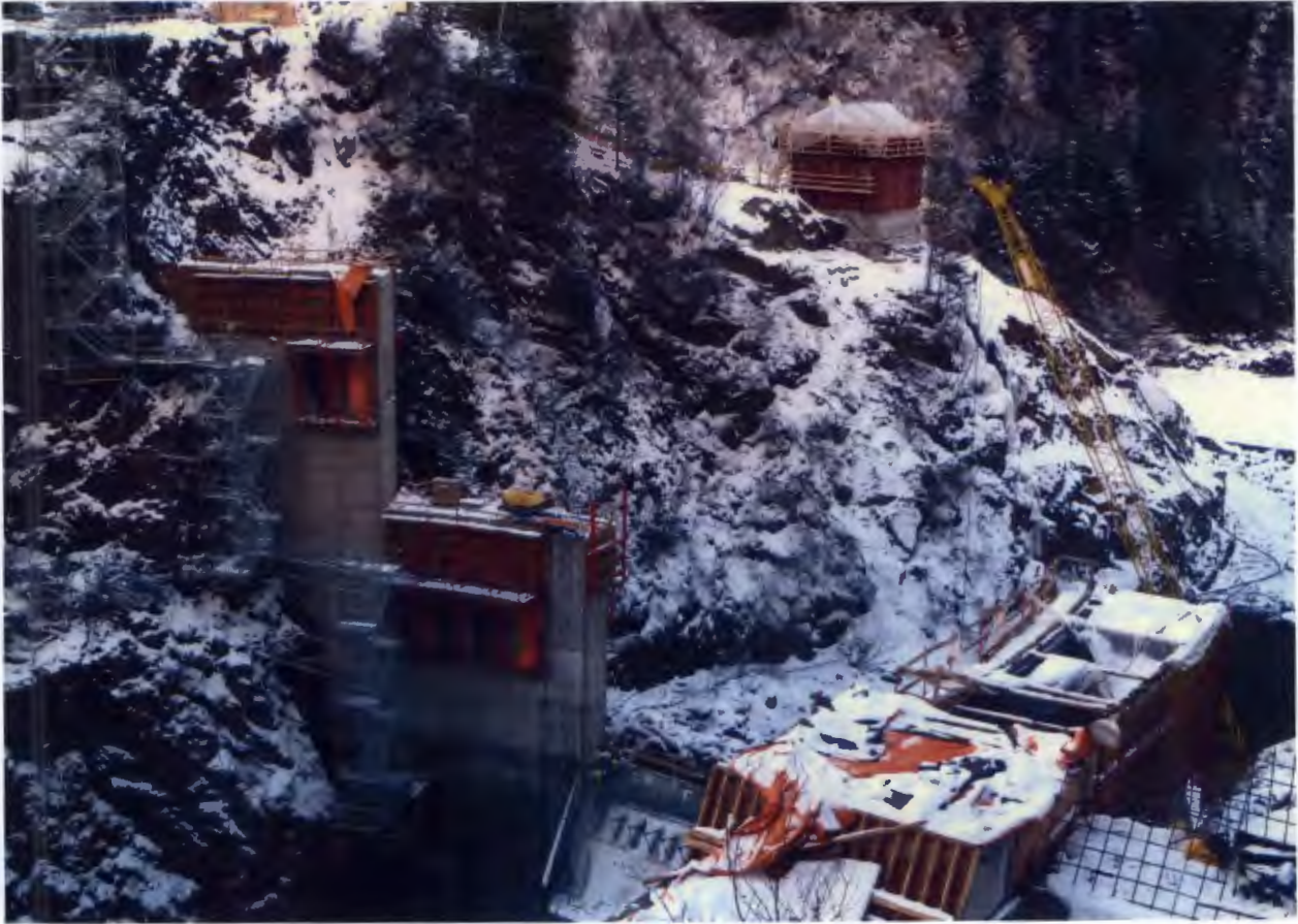
Figure 3. Intake Portal and Right Abutment, Barnard completed forms for last placement of gatehouse wall.
