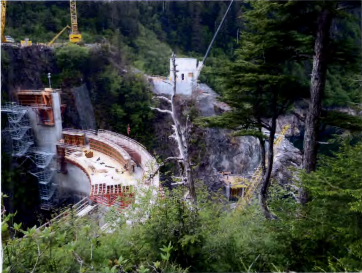
Figure 3. Intake Portal and Right Abutment, Barnard has tested the fit of the fixed wheel gate and will completed the intake structure June 4 as planned.
