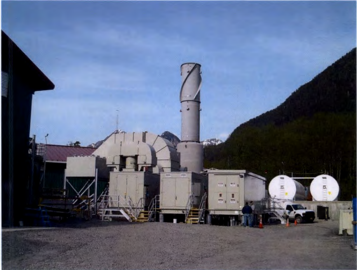
Figure 1. Titan 130 Diesel Turbine
