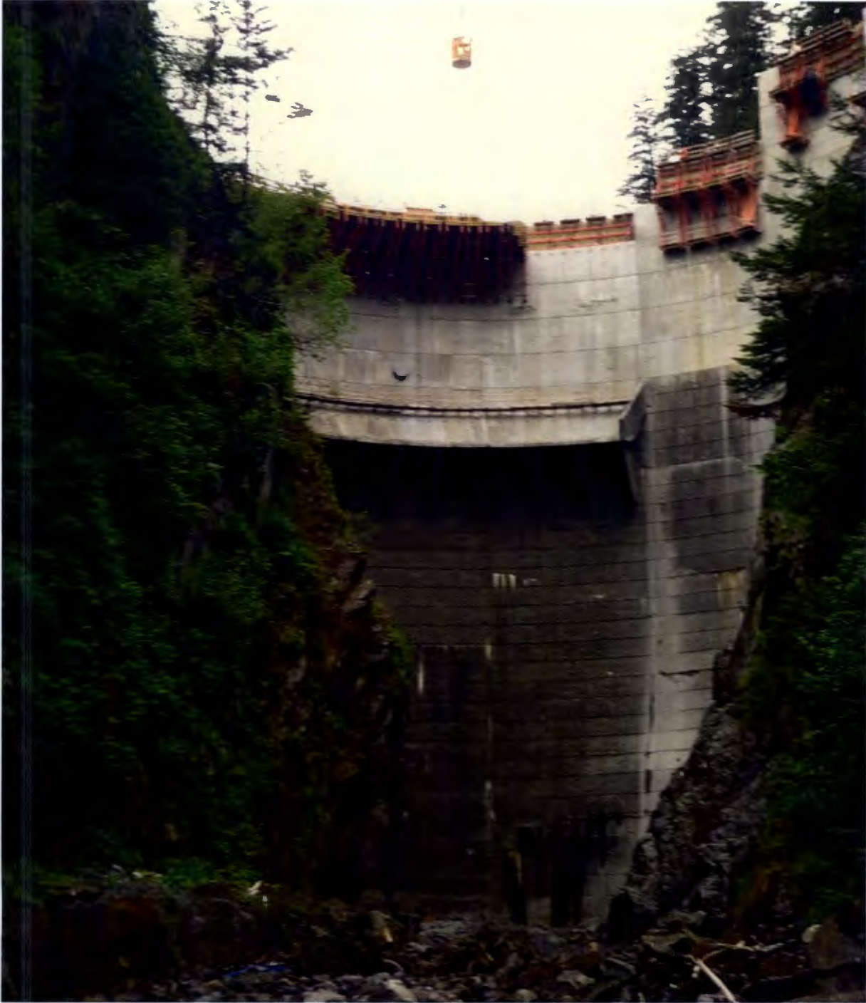
Figure 2. Drainage Tunnel and Scour Wall, Crux Subsurface (Crux) began working night shift on the dam curtain grouting and completed 3 holes on the right abutment. There will be a total of at least 9 holes on the right abutment and 17 holes on the left abutment. No geological surprises have been discovered, however, the contractor has had difficulty with the drilling.
