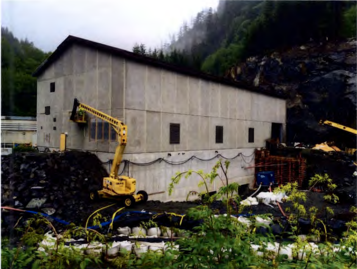
Figure 7. Powerhouse Site, NAES has completed the installation of conduit and cable tray in and outside the powerhouse. AMCL placed forms for the raw water intake.
