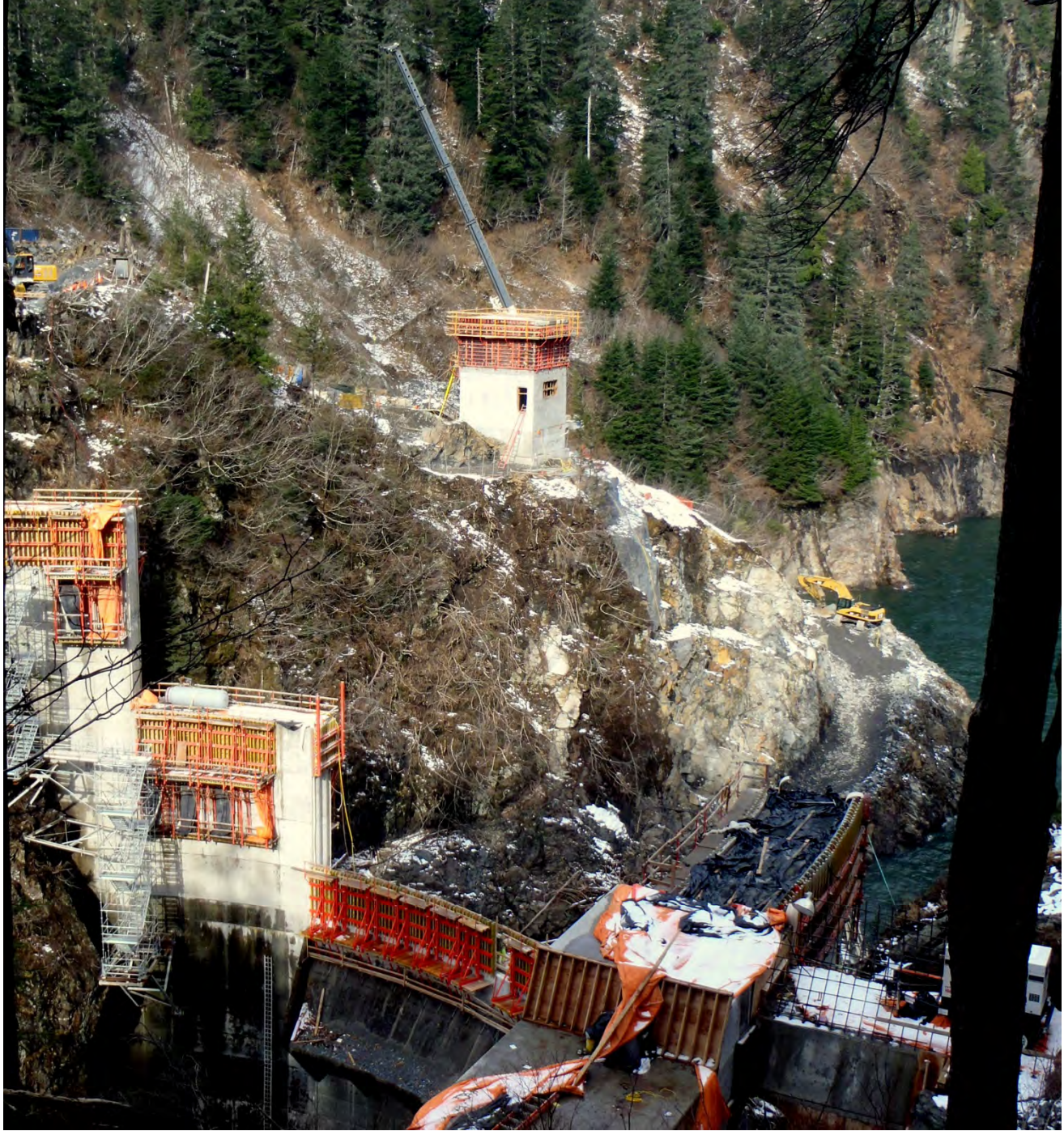
Figure 3. Intake Portal and Right Abutment, Barnard scaled intake portal to completed intake portal excavation.
