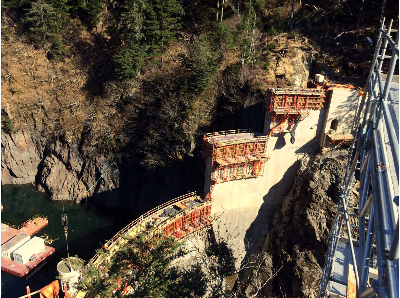
Figure 1. Dam and Left Abutment Area, Barnard made final concrete placement on dam keyway and began forming for dam raise blocks M3-M5 (in the old spillway).
