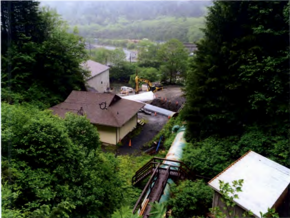
Figure 6. Lower Portal Area, Barnard placed CDF around the new penstock from the turbine inlet pipes up to the water treatment plant access road.
