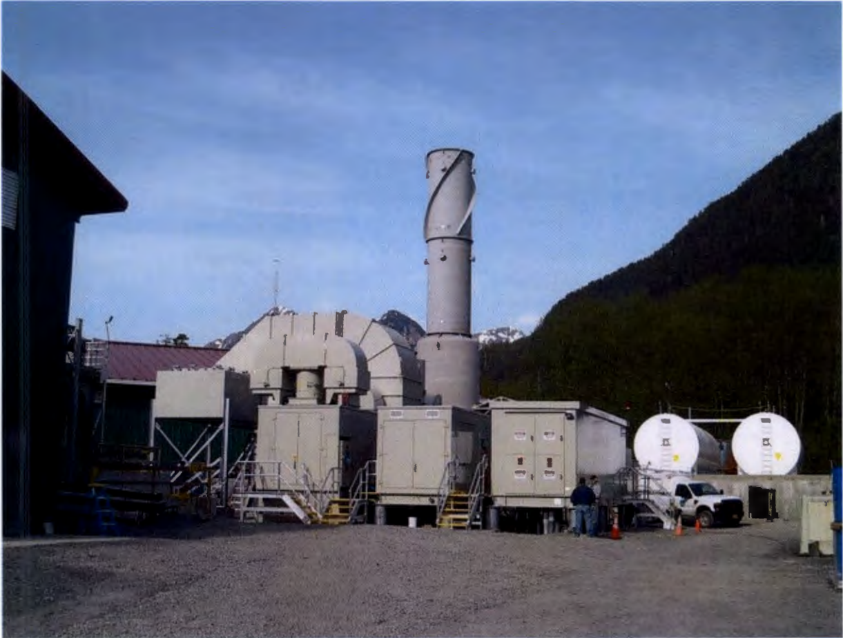
Figure 1. Titan 130 Diesel Turbine
