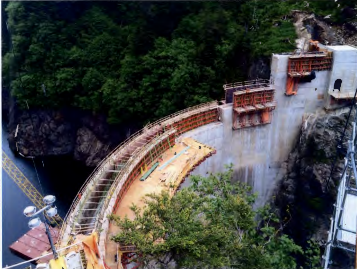
Figure 1. Dam and Left Abutment Area, Barnard began erecting the spillway form support structure for the dam spillway construction. Barnard showed good progress on the dam construction completing 6 block placements
