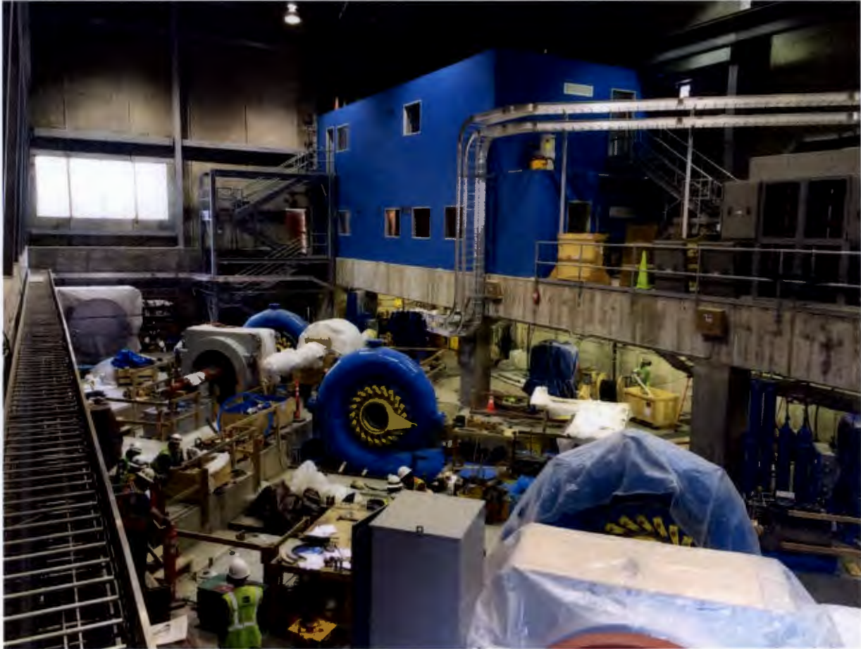
Figure 8. Powerhouse Interior, NAES performed the following tasks related to the turbine generator installation: completed secondary concrete placement around draft tubes, completed alignment of all 3 turbine spiral cases, installed all inlet valves and welded all turbine inlet pipes to the penstocks, completed alignment of all generator sole plates, located all Turbine generator control panels in powerhouse, moved all stators and rotors to powerhouse, completed alignment of generator, bearings, exciter and runner in BL3, and modified BL5 bearing pedestals to correct error in the soleplate alignment. NAES also completed the installation of the low voltage and medium voltage switchgear in the powerhouse.
