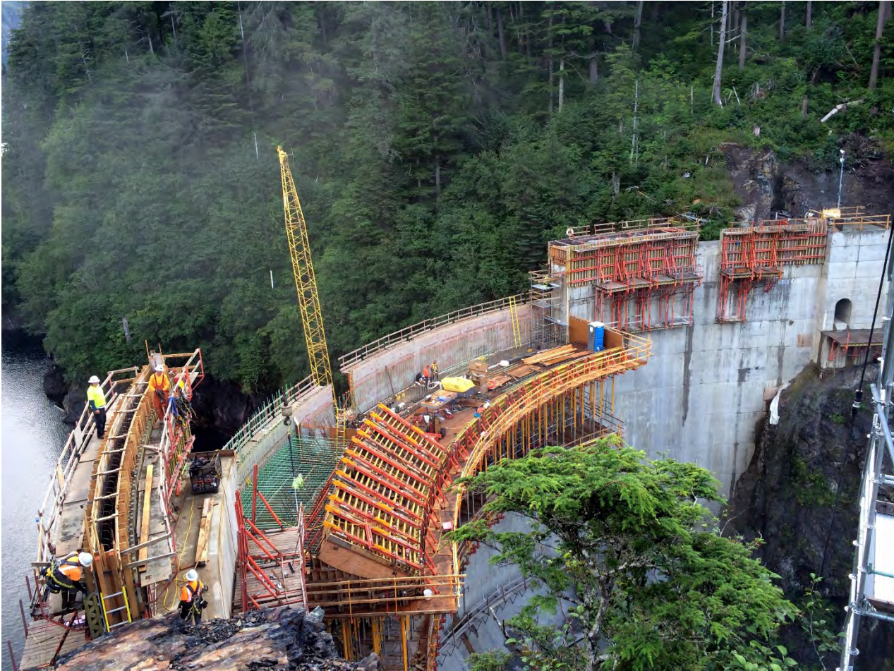
Figure 1. Dam and Left Abutment Area, Barnard showed good progress on the dam construction completing 2 block placements . TO DATE – 53 of 53 blocks placed on the Dam Raise. In June Barnard started work on the spillway section of the dam, which is the most complicated formwork for the dam raise. Eight of 9 placements completed on the Left Abutment and Cutoff Wall. Crux completed all curtain grout holes on the left abutment.
