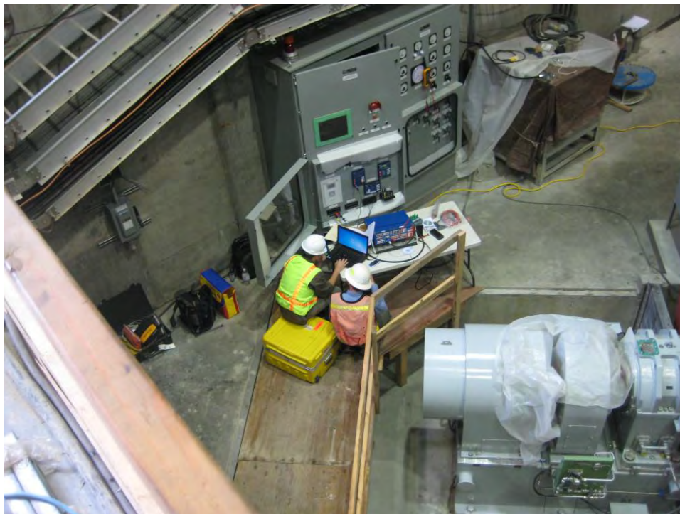
Figure 7: Dry Commissioning Unit #3 Turbine Control Cabinet
