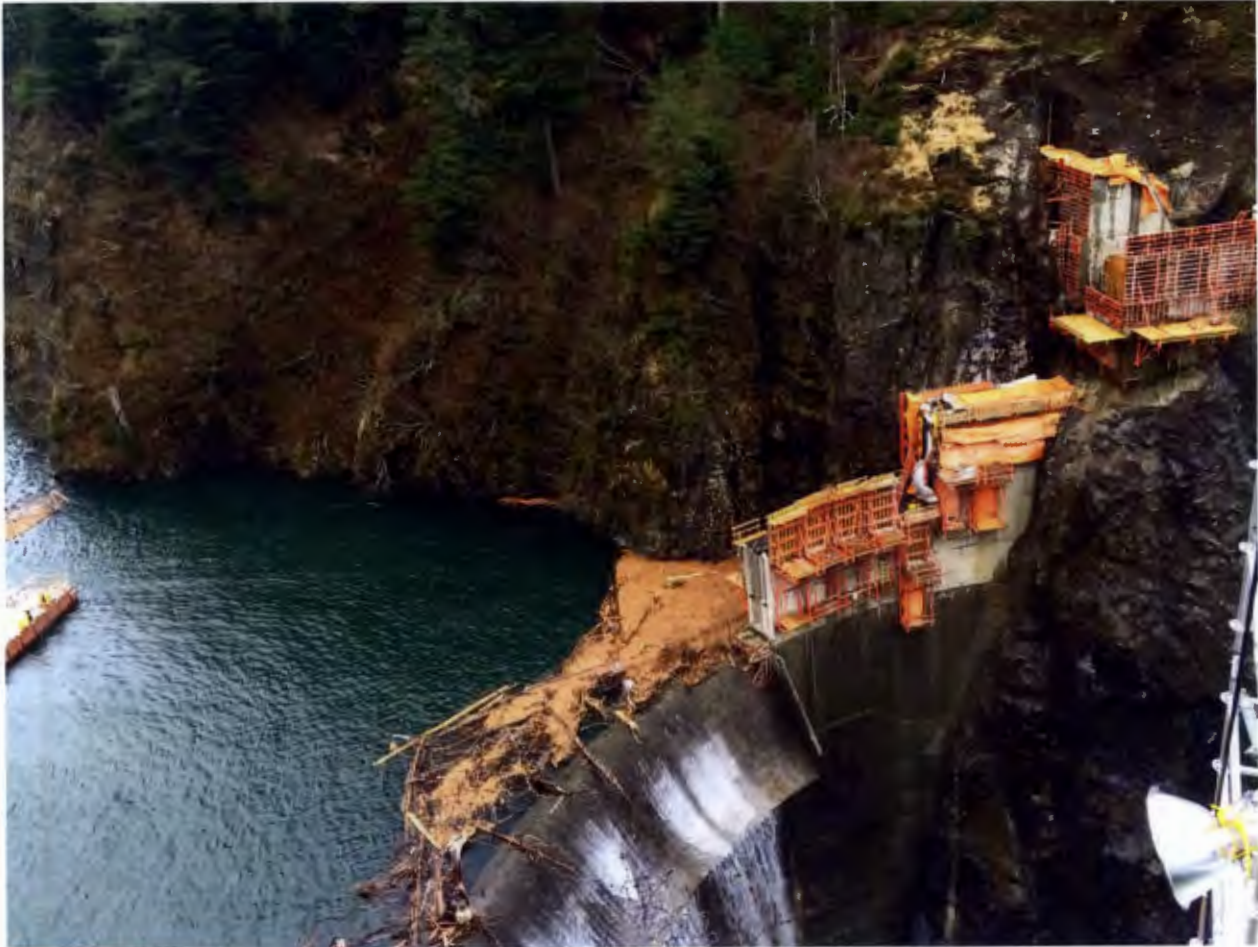
Figure 1. Dam and Left Abutment Area, Barnard made 1 concrete placement at the thrust block, 1 placement at the cutoff wall, and 3 block placements in the main dam near the left abutment.
