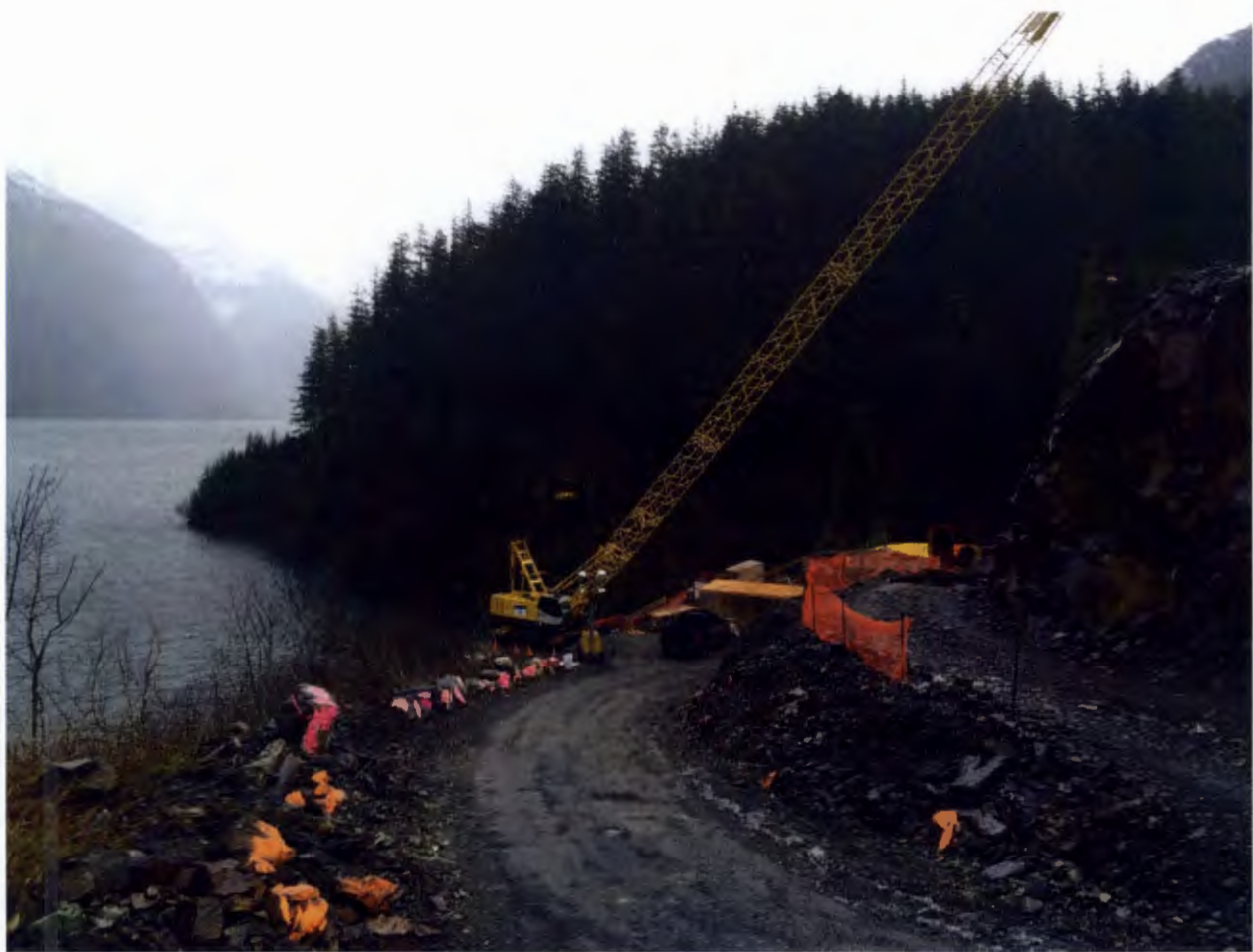
Figure 4. Gate House Location, Barnard made 2 placements at the gate shaft and 2 placements remain.
