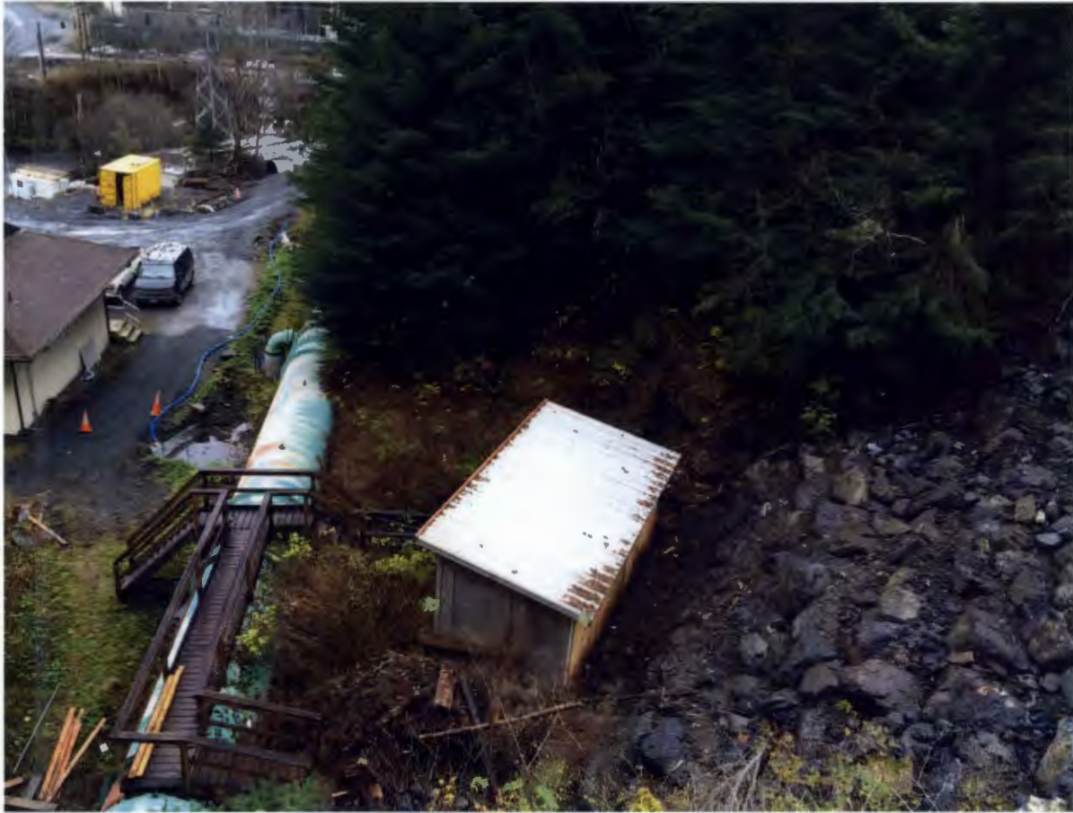
Figure 6. Lower Portal Area, Barnard completed replacing the timber crib wall at the lower portal with rock.
