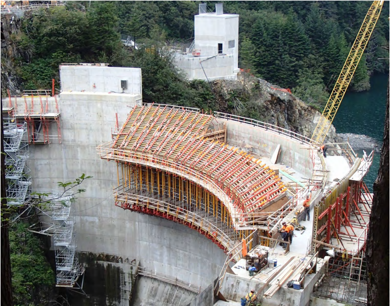
Figure 2. Intake Portal and Right Abutment, Blue Lake Tunnelers completed the excavation of both tunnel tie-ins. Barnard began forming the tunnel plug that will seal off the existing intake.
