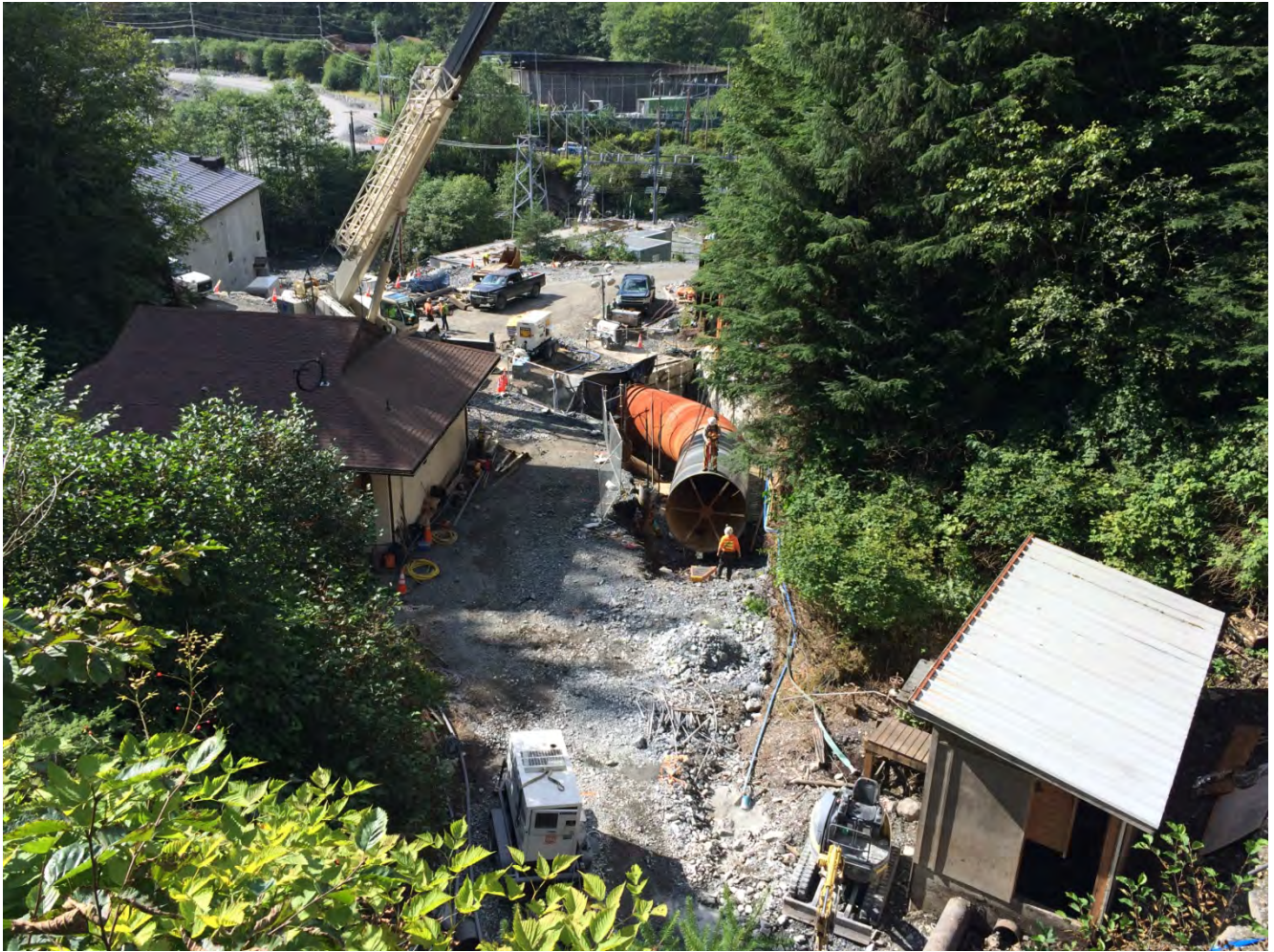
Figure 6. Lower Portal Area, The lower portal penstock was removed and installation of the new penstock continued.
