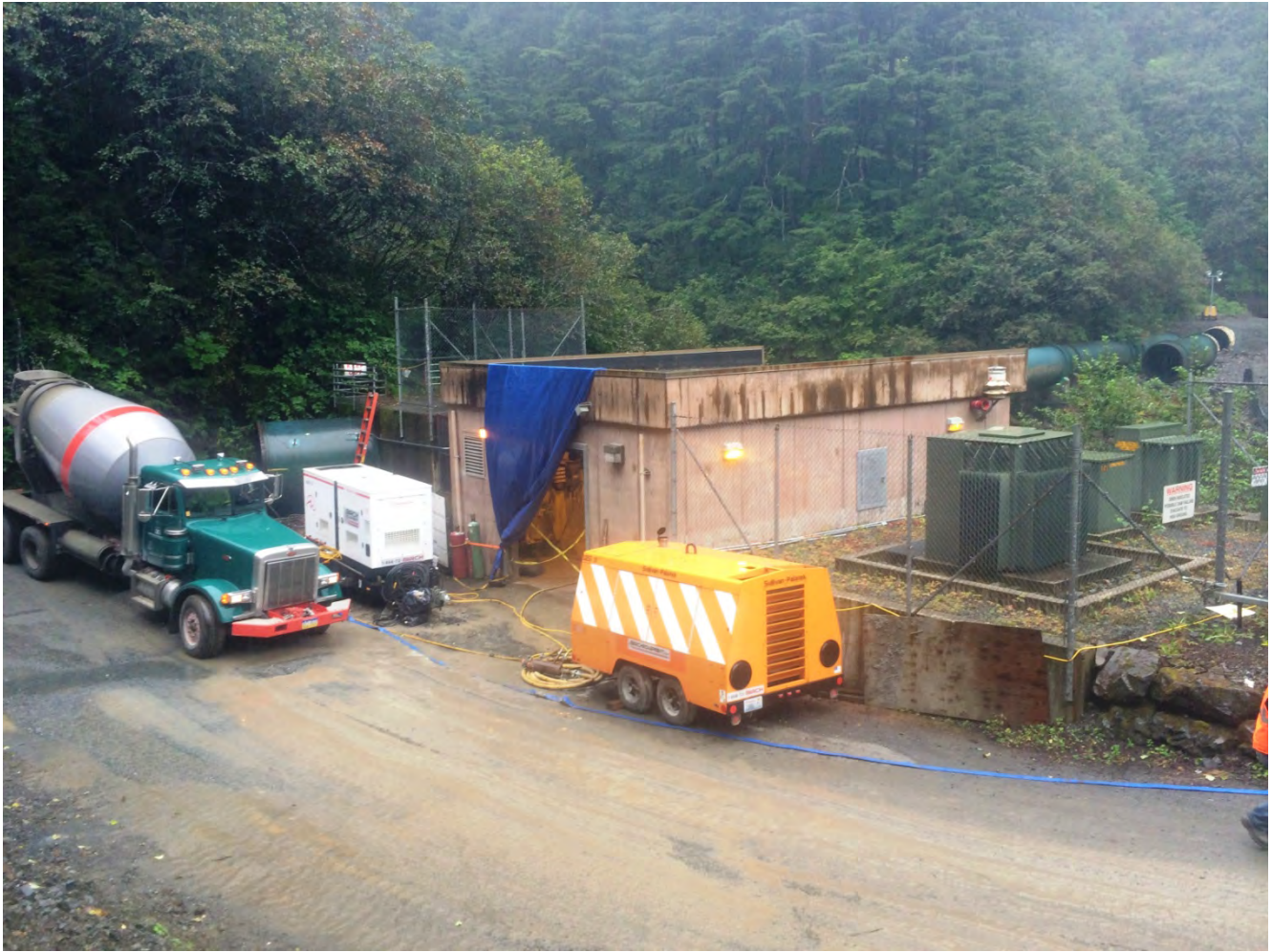
Figure 5. Fish Valve Unit and Upper Portals, Barnard completed the installation and grouting of the tunnel south portal steel liner. The existing FVU turbine-generator was completely removed from the FVU powerhouse building.
