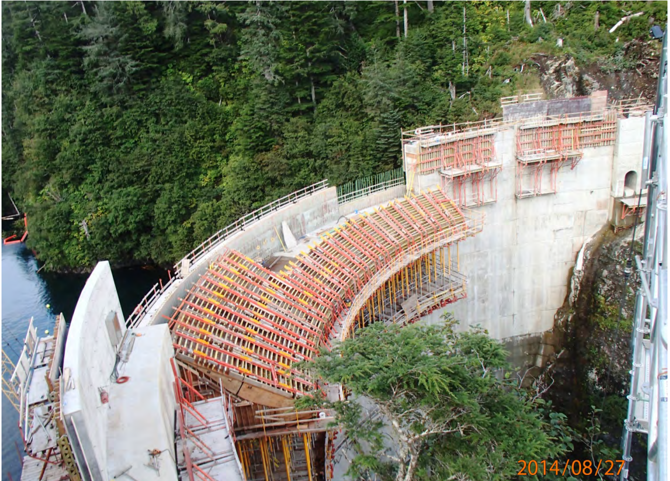
Figure 1. Dam and Left Abutment Area, Crux completed the curtain grouting at the dam. Barnard crews completed 7 major concrete placements on the dam, including M3/410 and 417, M4/410, M5/410, M2 parapet wall, M6 crest slab and M7 crest slab.
