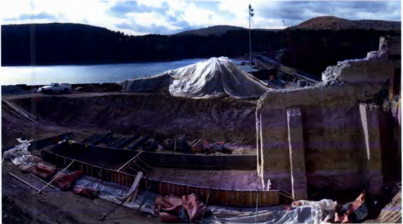
At Gilboa Dam, crews are now reconstructing the east training wall's two upstream monoliths.
