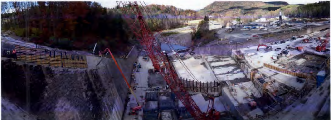
Reconstruction of the top of the west training wall progresses from within the plunge pool.
