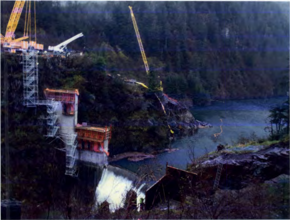
Figure 3. Intake Portal and Right Abutment, Barnard has completed 14 of 79 blocks of concrete at the dam. The blocks on the right abutment are now up to El 425.
