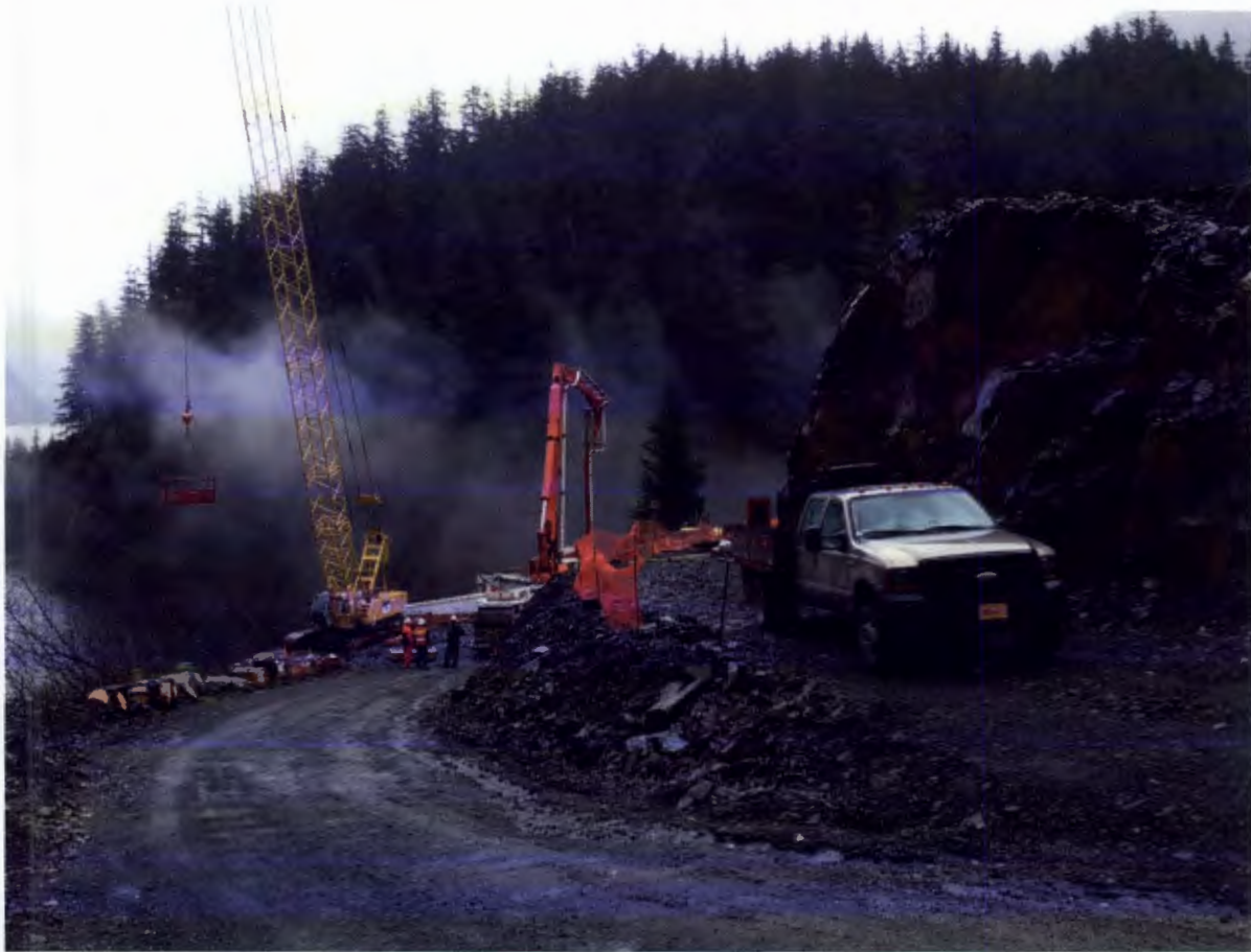
Figure 4. Gate House Location, Barnard formed and placed concrete in the gate chamber crown and in the intake gate shaft.
