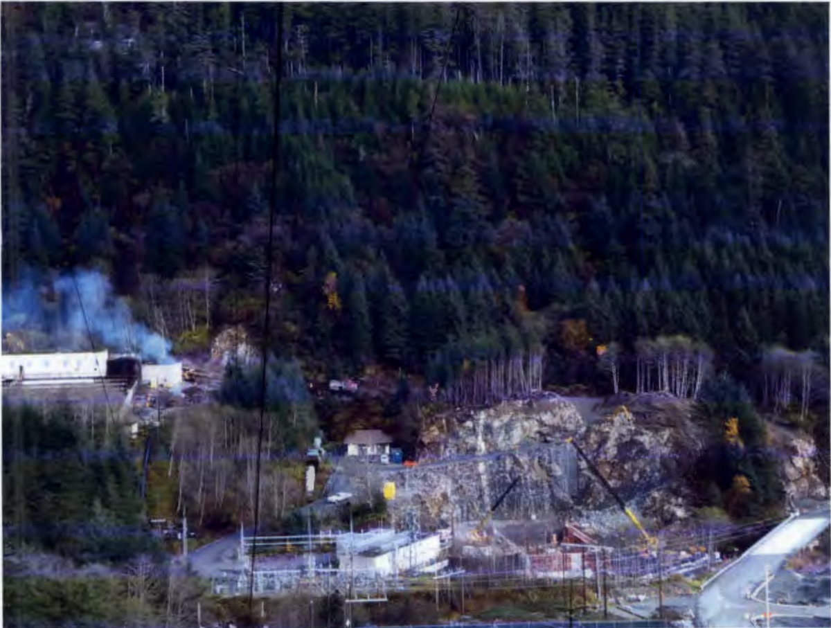
Figure 9. Lower Project Site, Removal of the rock knob at the powerhouse access road continues.
