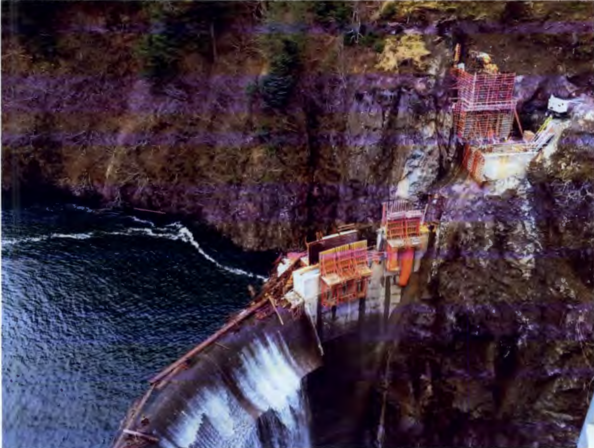
Figure 1. Dam and Left Abutment Area, Barnard made the first concrete placement on both the left abutment thrust block and cutoff wall.
