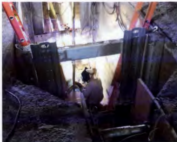
Newly installed pipe is tied-in at the L-220 Project in Davis, California.
