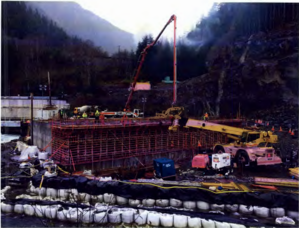
Figure 7. Powerhouse Site, ASRC McGraw Constructors (AMCL) placed 221 CY of concrete at the north and west walls and 170 CY at the south and west walls of the powerhouse. To date 2800 CY of 3350 CY have been placed at the powerhouse.
