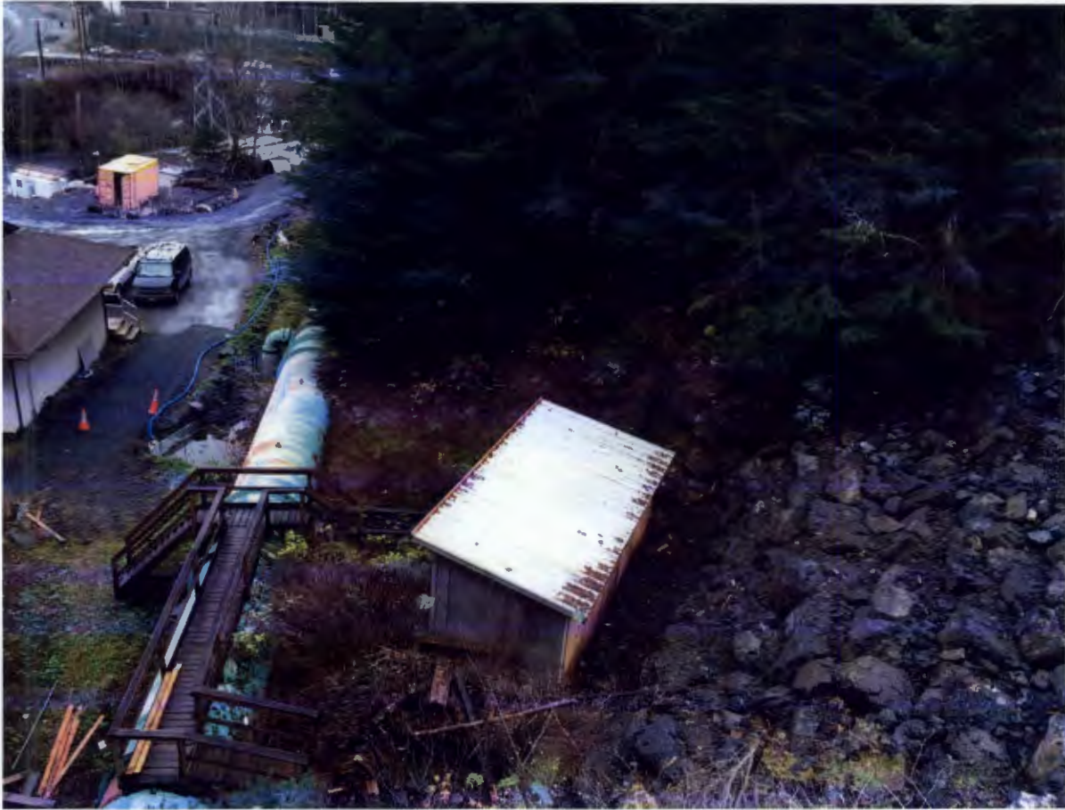
Figure 6. Lower Portal Area, Barnard completed replacing the timber crib wall at the lower portal with rock.
