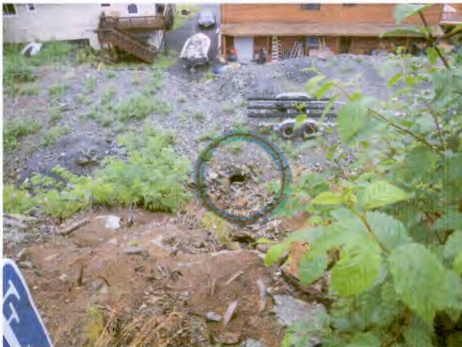
CBS has inherited maintenance responsibility for numerous drainage structures to which we do not have physical access. This reality makes it difficult if not impossible to properly maintain. When culverts like this one gets plugged and can't be accessed for maintenance, and if private property is flooded as a result, there could be legal consequences (Hillside Subdivision, 2012).
