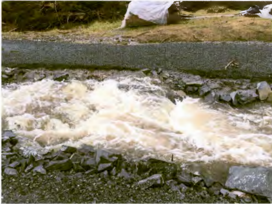
The runoff generated from this storm flowed over the top of the ditch and eroded portions of the adjacent trail. Riprap ditch liner was too small and washed down the ditch. This situation is fairly common throughout Sitka (Benchlands 4-lot Subdivision, 2015).
