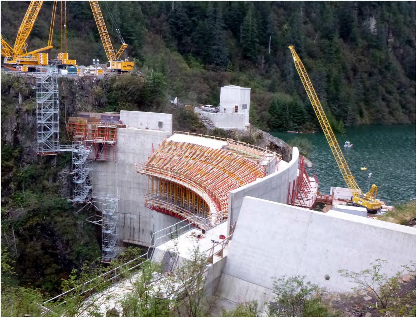
Figure 2. Intake Portal and Right Abutment, The concrete tunnel plug was completed in the existing intake tunnel. Tunnel and penstock were closed up in preparation for filling.
