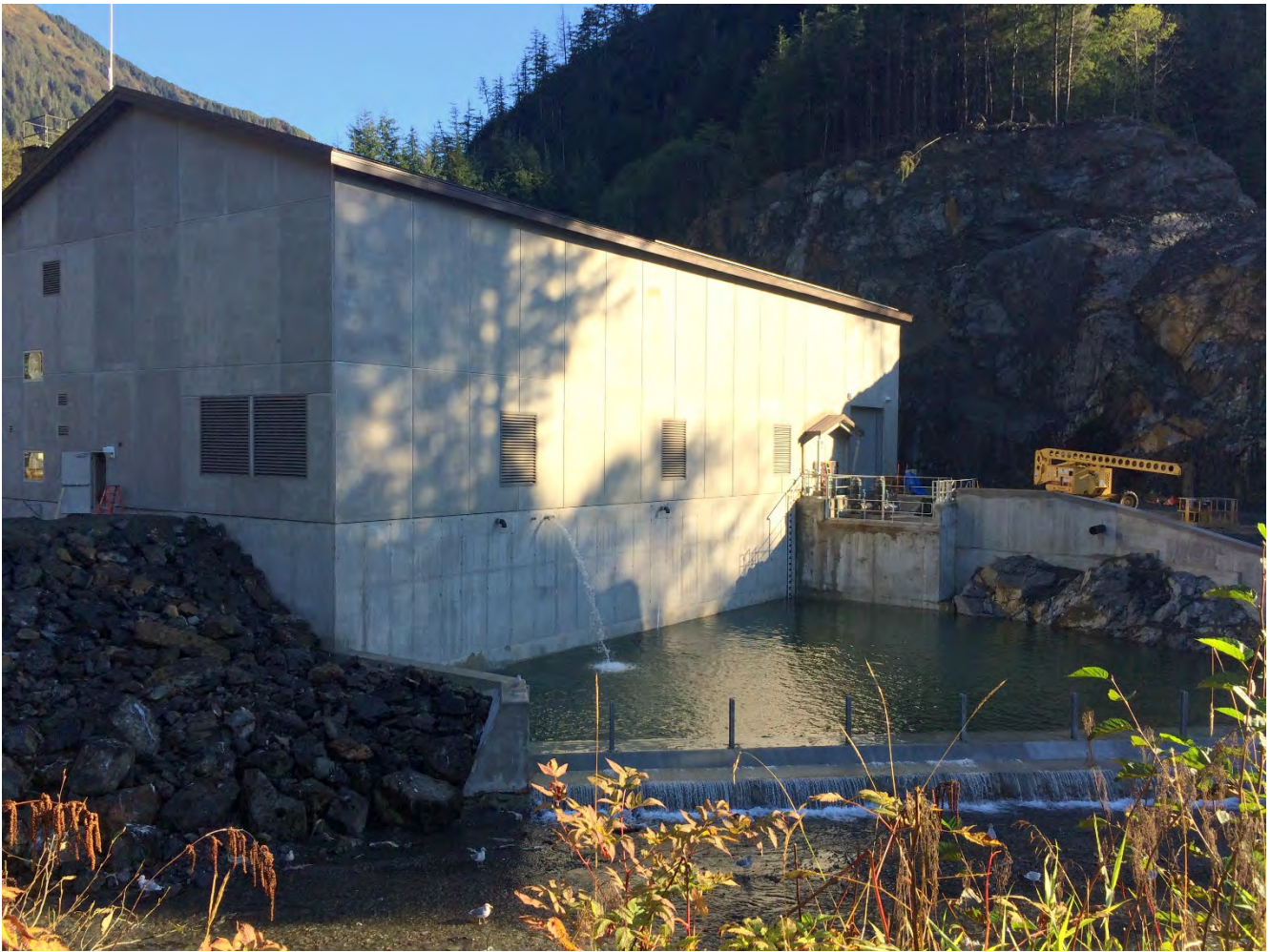
Figure 6. Powerhouse Site, ASRC continued to build out the service and raw water systems.
