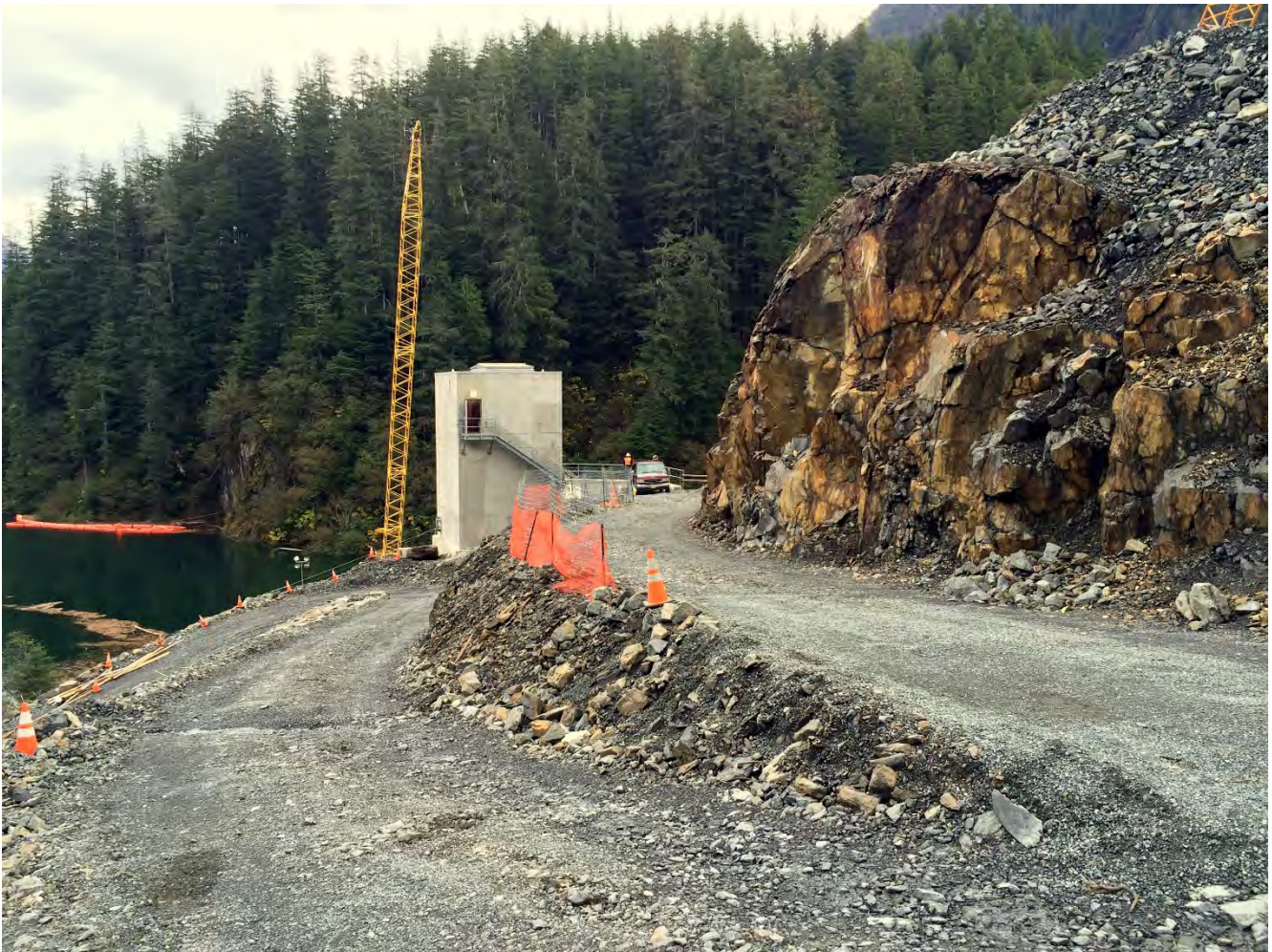
Figure 3. Gate House Location, Began flushing and rock removal from upper tunnel by opening a valve on the bulkhead gate and opening the fixed wheel gate. The bulkhead gate was later removed for filling of the tunnel.
