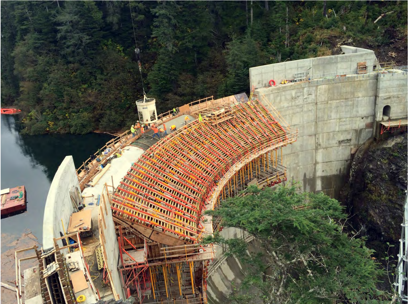
Figure 1. Dam and Left Abutment Area, Barnard crews completed 8 major concrete placements on the dam, including M1 crest slab, M3/425, M4/417, and 425, M5/417, Cutoff wall to El 440, M6 parapet wall and M7 parapet wall.
