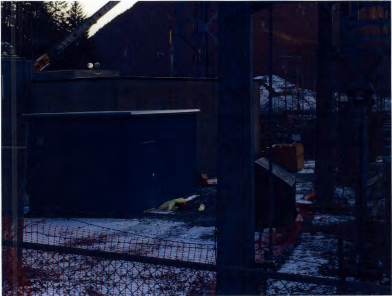
Additional Figure 9. Switchyard Control Building, John Rennie reached substantial completion on the switchyard control building.
