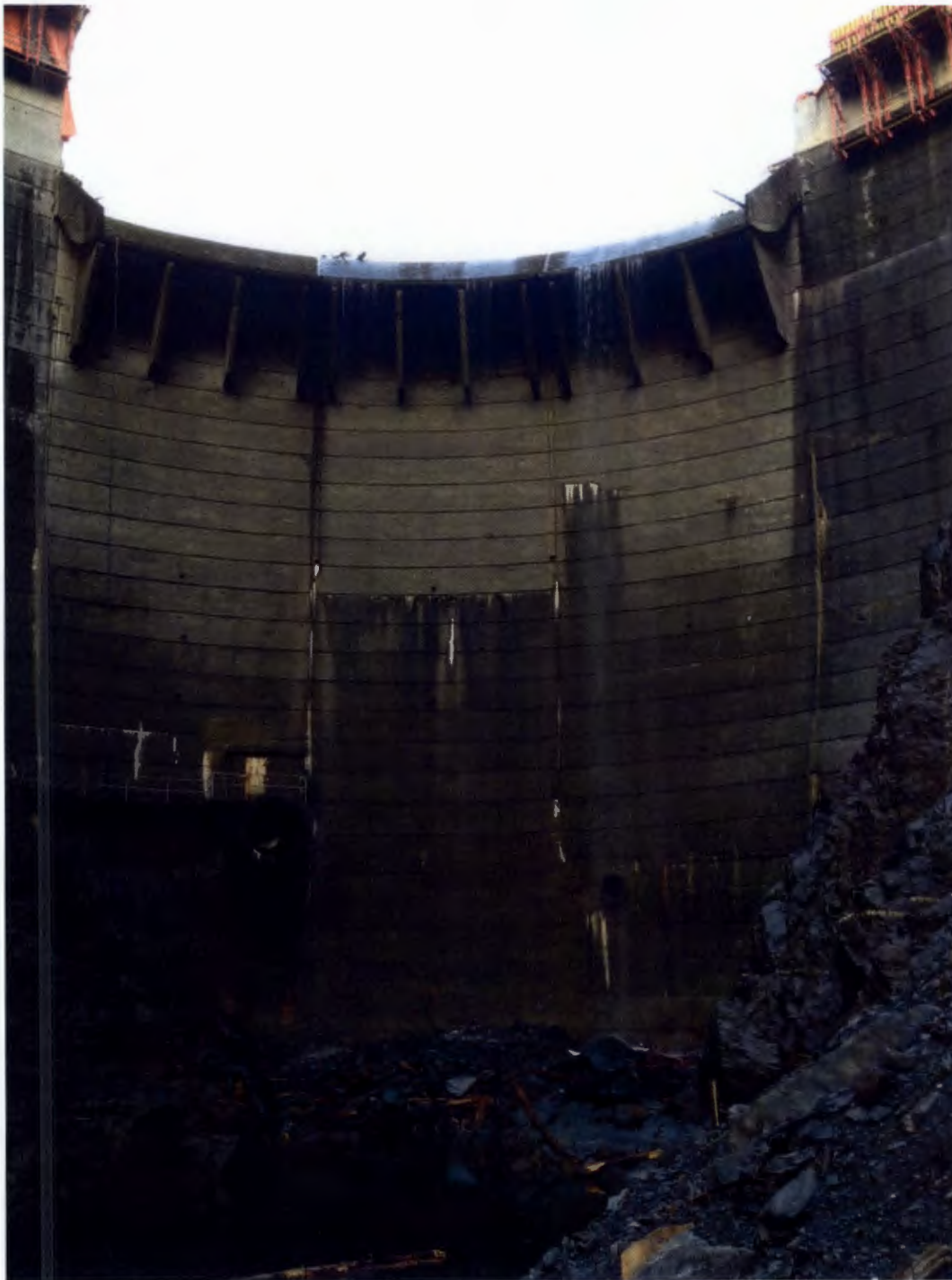
Figure 2. Drainage Tunnel and Scour Wall, The dam continued spill on and off through November.
