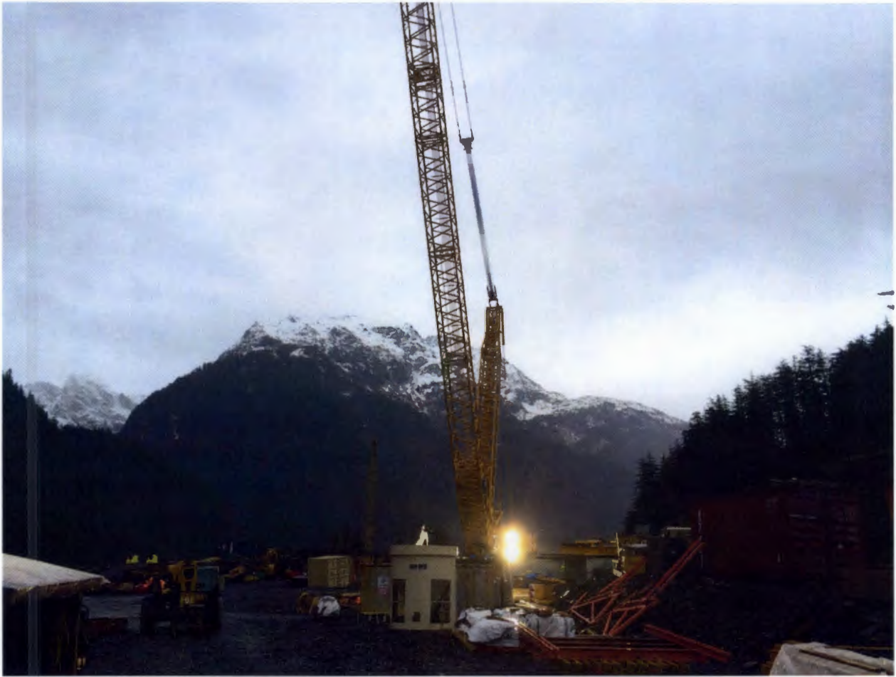
Figure 5. Dam Staging area, 9 days were lost at the dam site due to weather or winds shutting down the crane.
