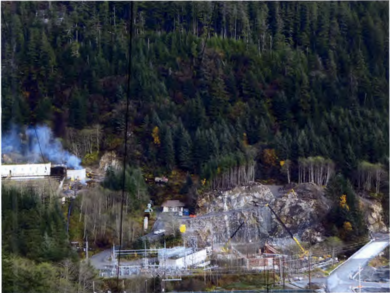
Figure 8. Lower Project Site, Removal of the rock knob at the powerhouse access road is complete.
