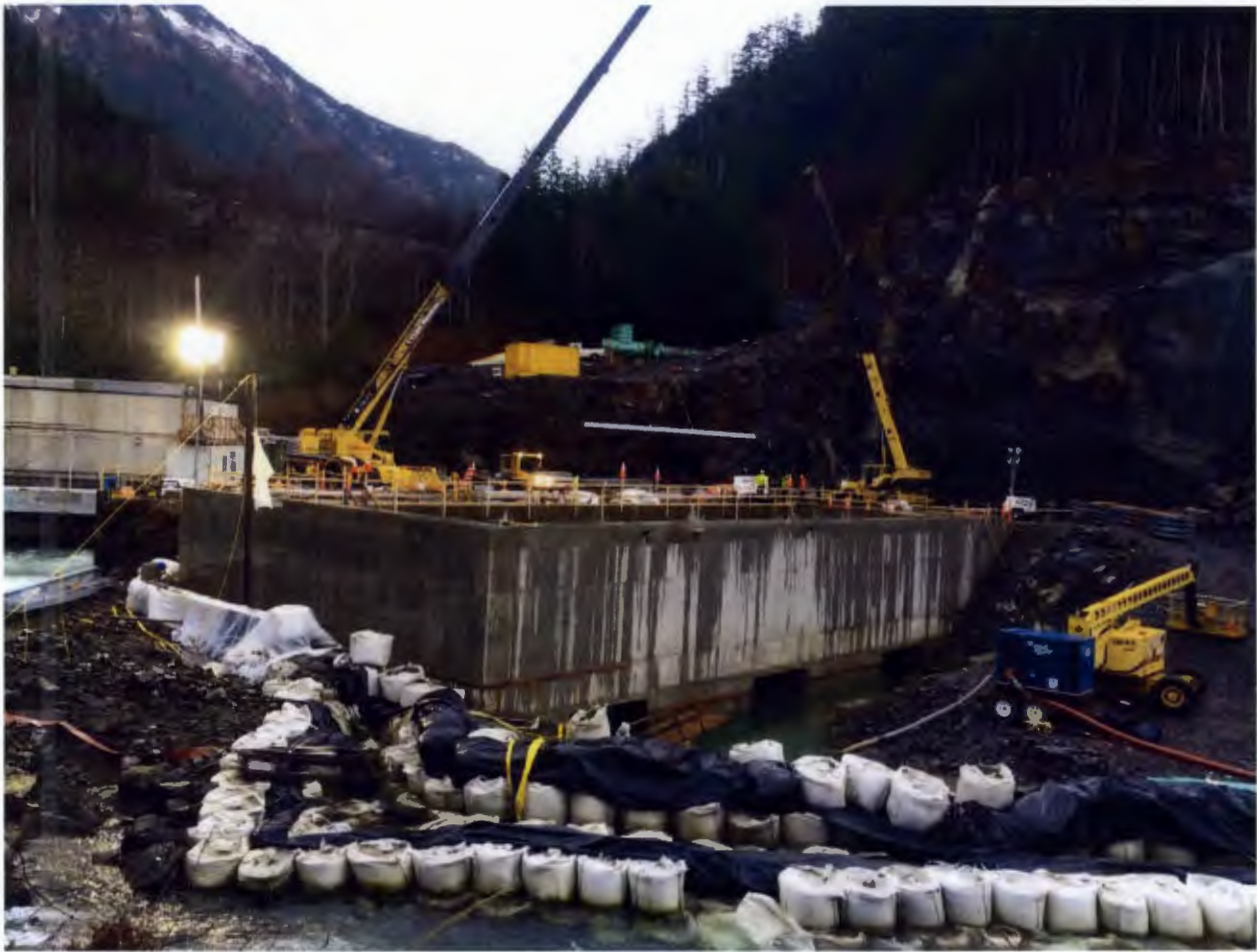
Figure 7. Powerhouse Site, ASRC McGraw Constructors (AMCL) placed 208 CY of concrete at the access bay rat slab, 99 CY at the mezzanine deck and 225 CY of concrete completing the el. 27 vehicle access deck. These placements substantially complete all primary concrete at the powerhouse site.
