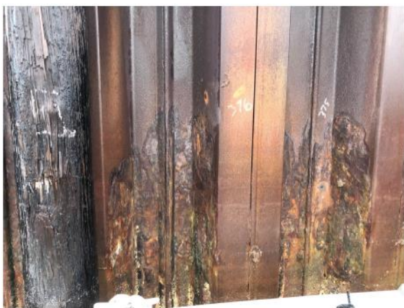
Figure 3- Sheet Pile Corrosion in Splash Zone, July 2021
