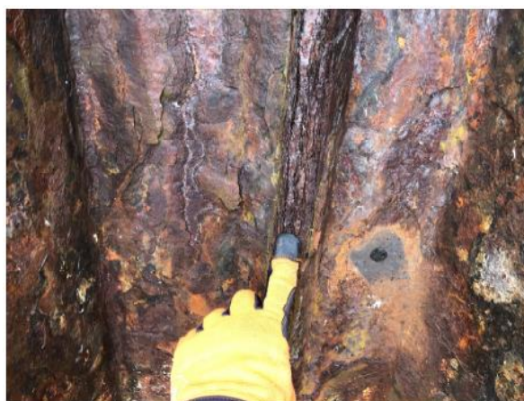
Figure 4- Sheet Pile Corrosion in Splash Zone, July 2021
