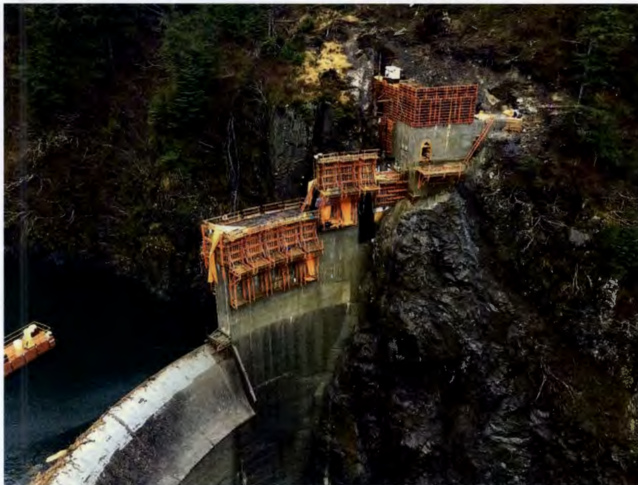
Figure 1. Dam and Left Abutment Area, Barnard made 1 concrete placement at the thrust block, 1 placement at the cutoff wall, and 3 block placements in the main dam near the left abutment. Barnard also prepped the spillway.
