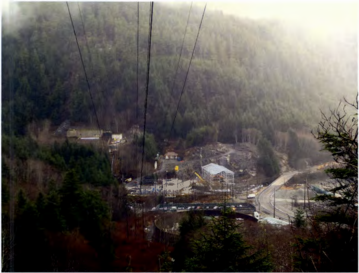
Figure 9. Lower Project Site, Southeast Earthmovers (SEEM) completed the access road excavation until rock bolting may be conducted.
